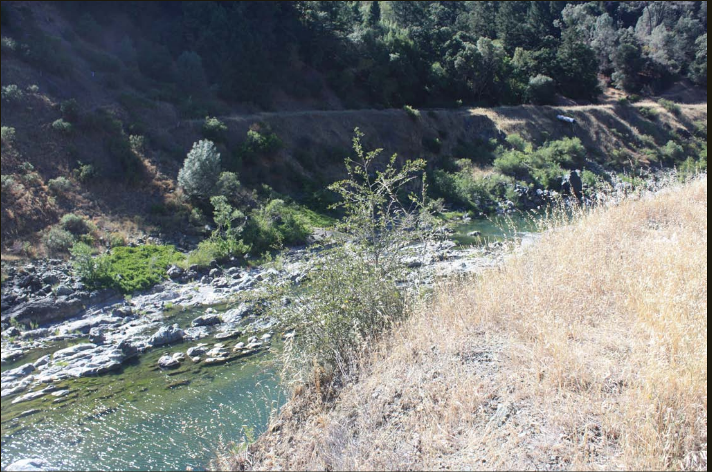
The SF&E/NWP grade along the Eel River, one mile south of Dos Rios. Note the grade is covered by a landslide in the left (south) part of the photo.
