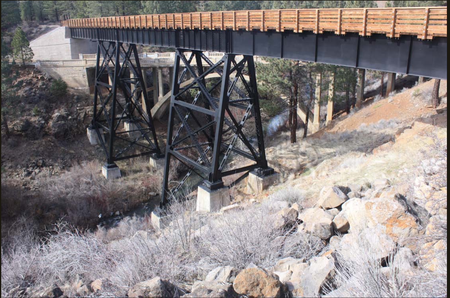
The Devil's Corral Trestle was built in 1913 to carry the F&L over a crossing of the Susan River, which the F&L followed almost the entire distance west of Susanville to Westwood. The eastern (near) 90 feet of the trestle was originally wood, but that was destroyed by a wildfire in 2000; in 2010 it was rebuilt as an entirely steel trestle for the Bizz Johnson Trail.
