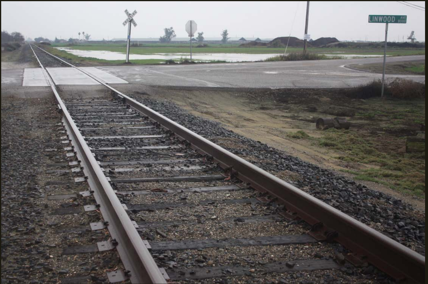
Southwestward view of the TS (1917) Hilmar Branch, same location as previous (one mile south of Hatch).
