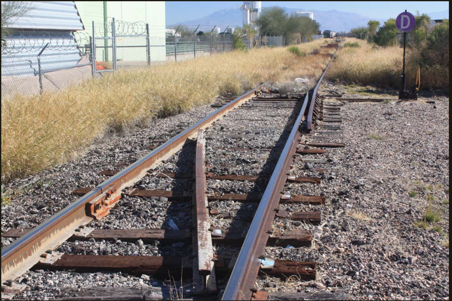
Eastward view of the industrial spur, which extends a half mile east of the SP (1881)/EP&SW (1912) mainline. The spur leads to the Cemex-Tucson facility, where the cylindrical tanks are visible to the left of the store cars. The line is clearly not in service; note the derail ("D") switch.
