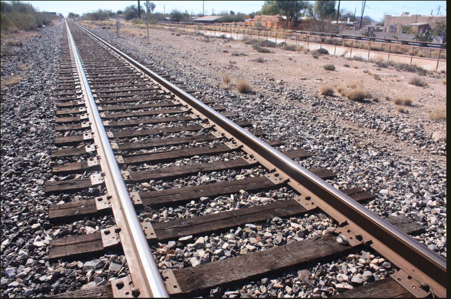
Southward view of the TB (1906) (T&N since 1910) at the same location as previous.
