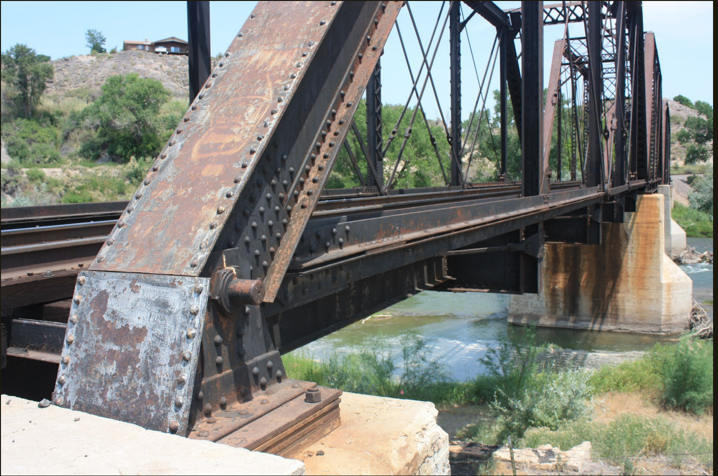
Northward view of the D&RGW North Fork Branch (1902n) 7.5 miles east of Delta, where a bridge carries the rails over the North Fork of the Gunnison River.
