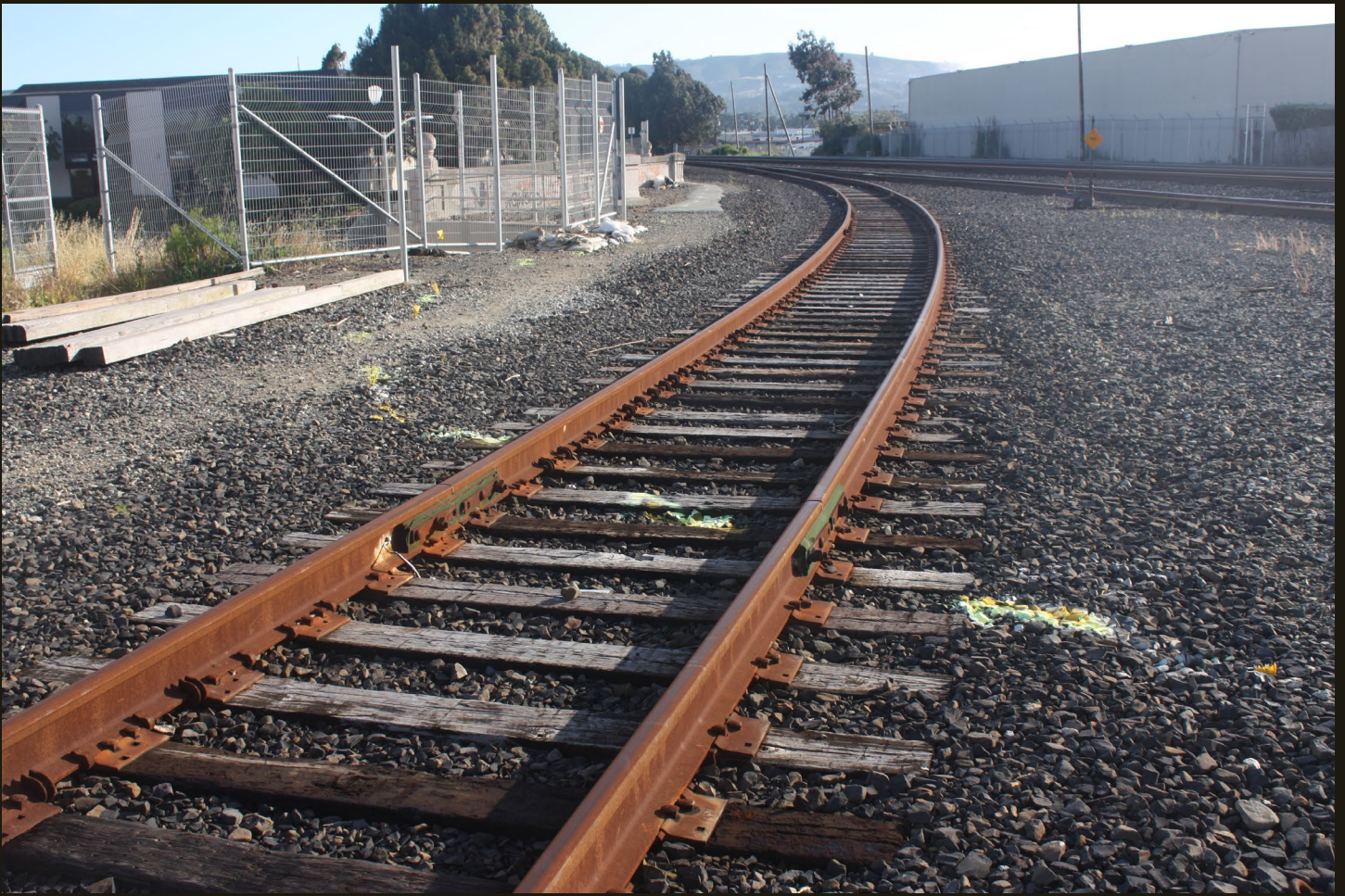
Southwestward view of the same rusty industrial spur off of the SP Monterey Line Bayshore Cutoff, a few steps east of the previous location. The spur once extended 1.5 miles east to San Bruno Point (on San Francisco Bay) but has been cut back about to about half that distance.
