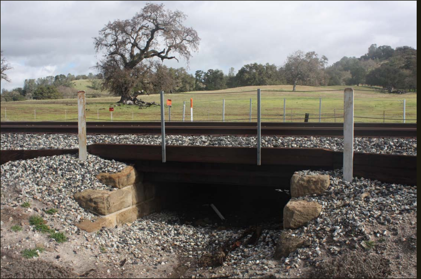
A nice masonry culvert on the SP (1894), 1 mile north of Santa Margarita.
