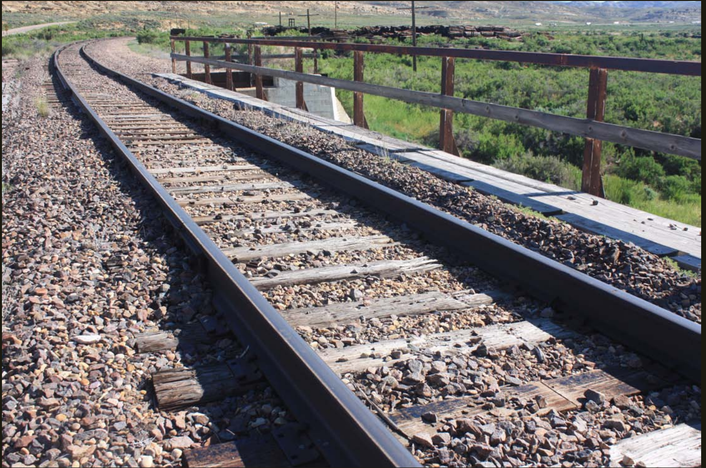
Northeastward view of the 1868 UP mainline around the Bitter Creek bend at Thayer Junction, northeast of the stored cars. Here the tracks curve eastward and join the active mainline 2 miles up (east). The bridge crosses the dry creek of Horsethief Canyon, which the UP Superior Branch followed up to the town of Superior.
