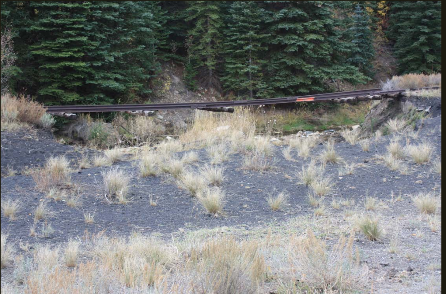
Washout along the U&PV grade.
