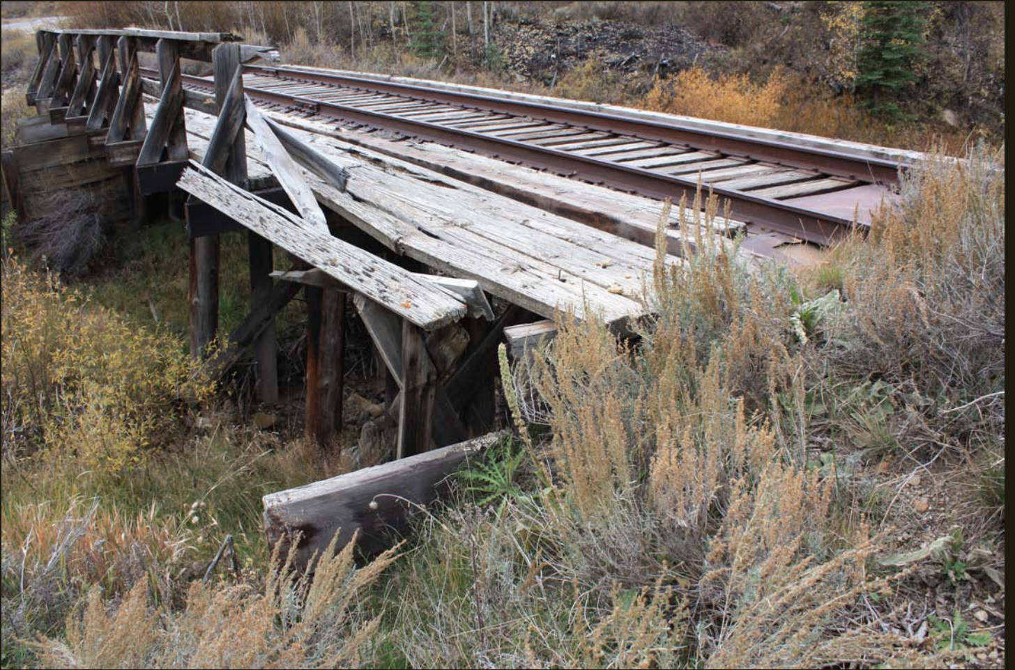
This crumbling bridge may be the original U&PV narrow gauge bridge built in 1879.
