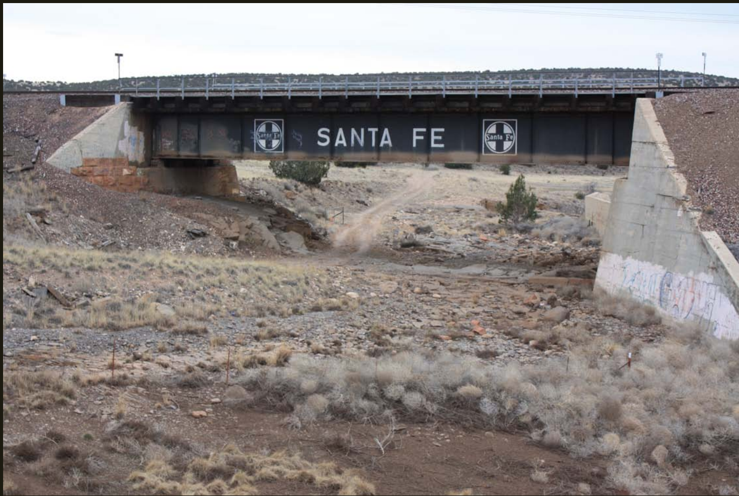
This AT&SF (now BNSF) bridge west of Ash fork has red Coconino Sandstone in the foundation. It is possible the sandstone is original A&P construction and the concrete is definitely later construction. However, both the sandstone and concrete are likely pre-1960, because similar bridge abutments are on the abandoned grade (see link east of this location).
