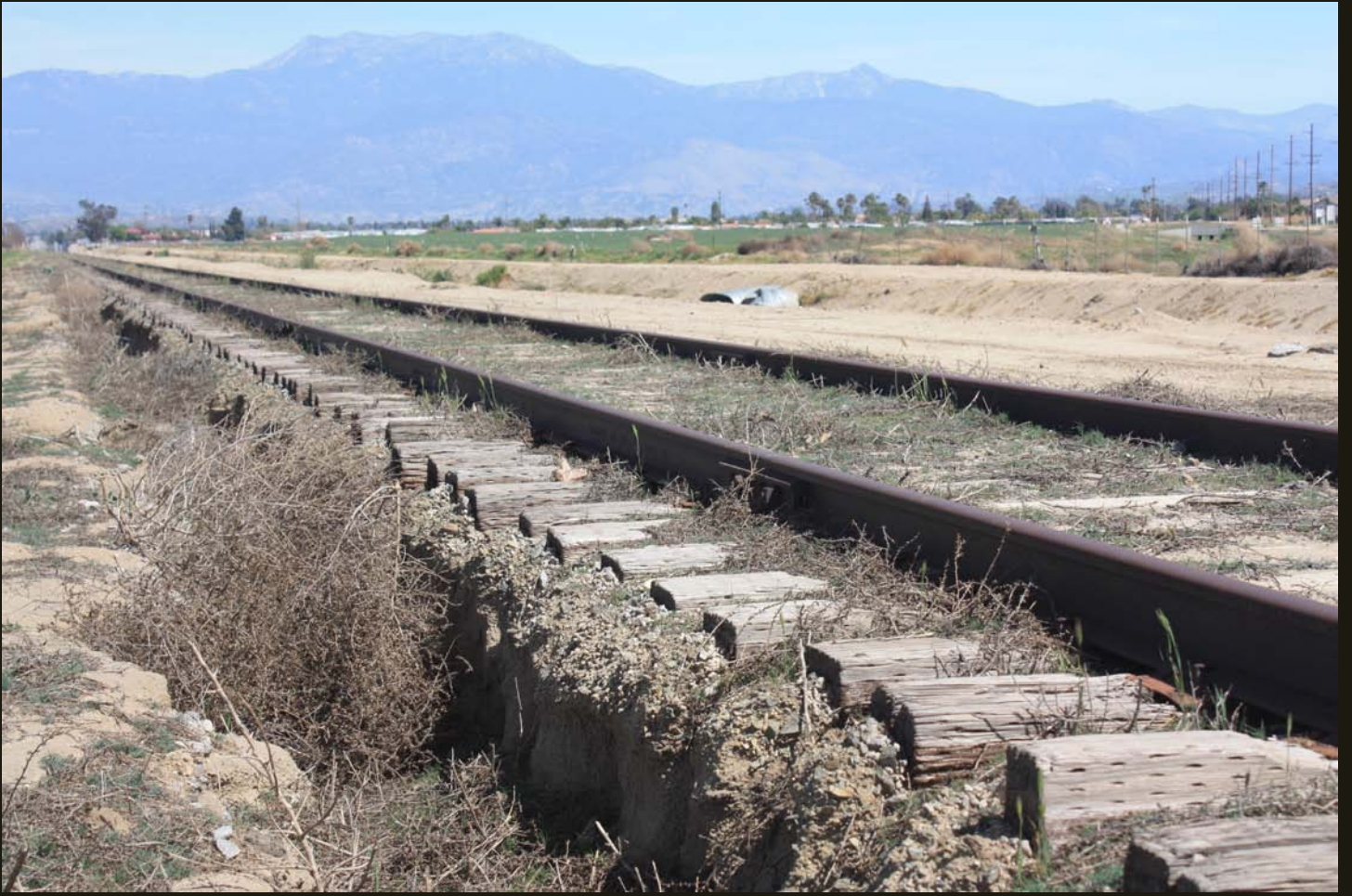
Same location as previous but two year later, after a washout.
