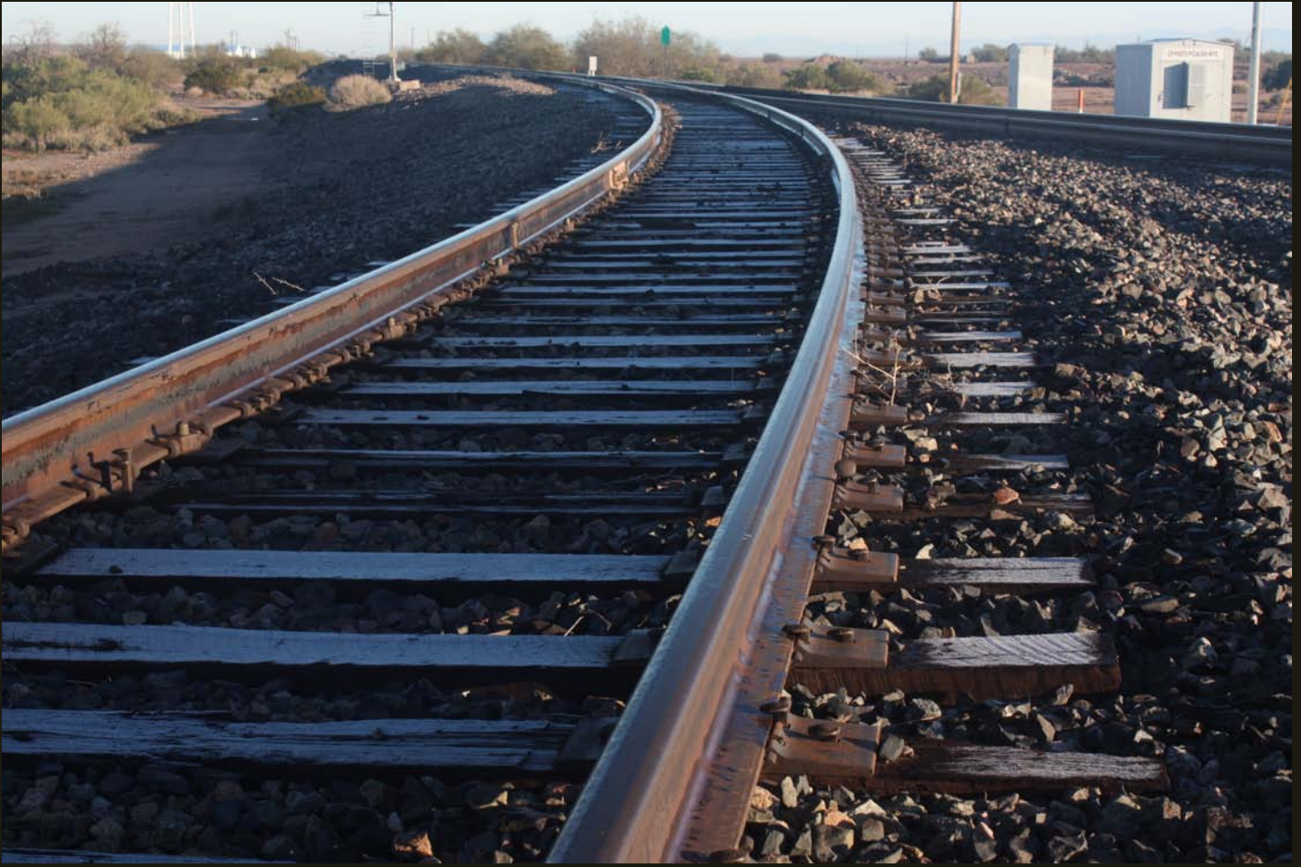
Northward view of the north tip of the of the Picacho wye, where the two branches of the wye converge to one track.
