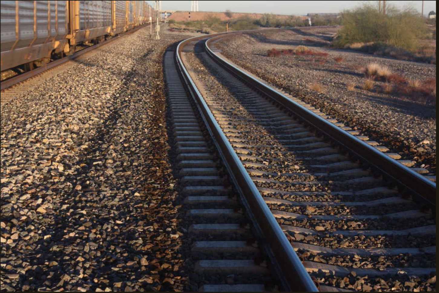
Northwestward view of the junction of the eastern branch of the Picacho wye. The junction for the western branch of the wye is barely visible in front of the bridge in the distance, which carries Arizona Highway 87 over the UP (former SP) mainline.
