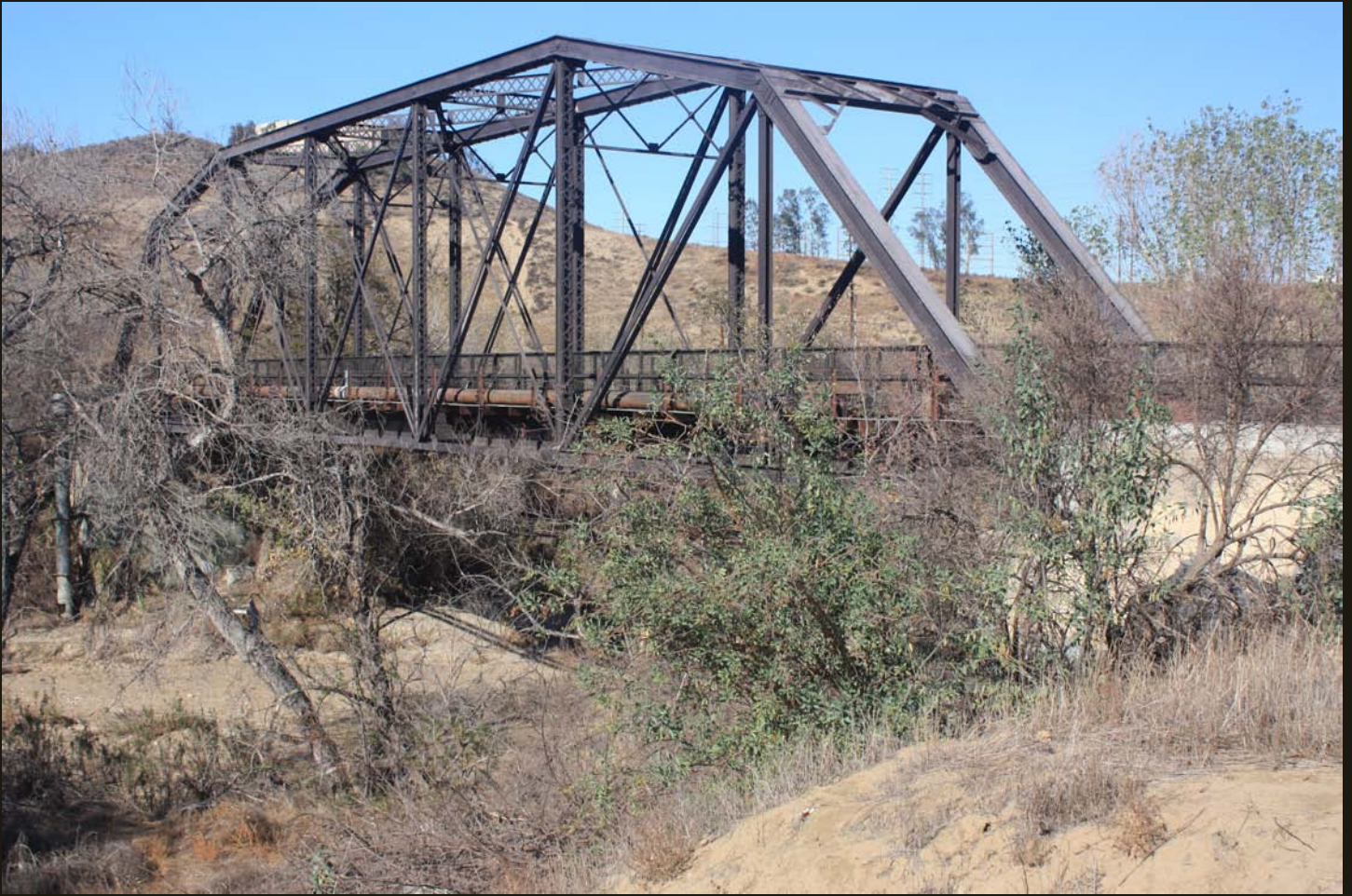
Another view of the Santa Clara River bridge, 2 miles west of the start of the SP (now UP) mainline.
