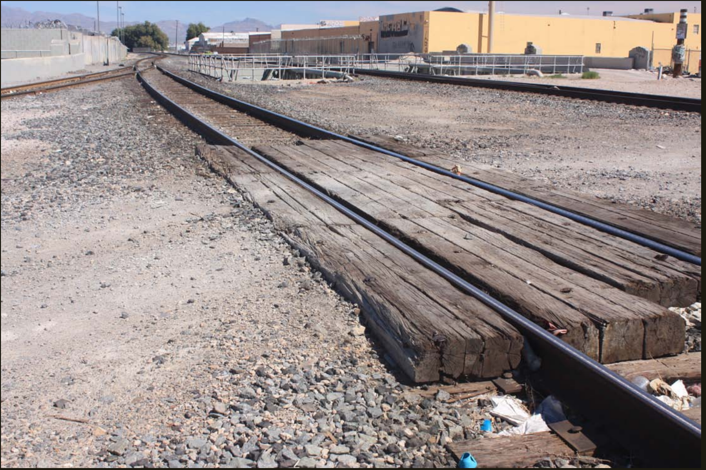
Northeastward view of the SPLA&SL (1905) a quarter mile northeast of the previous location. The mainline is on the right, the only remaining siding is in the foreground, and a rusty industrial spur heads to the left (west).
