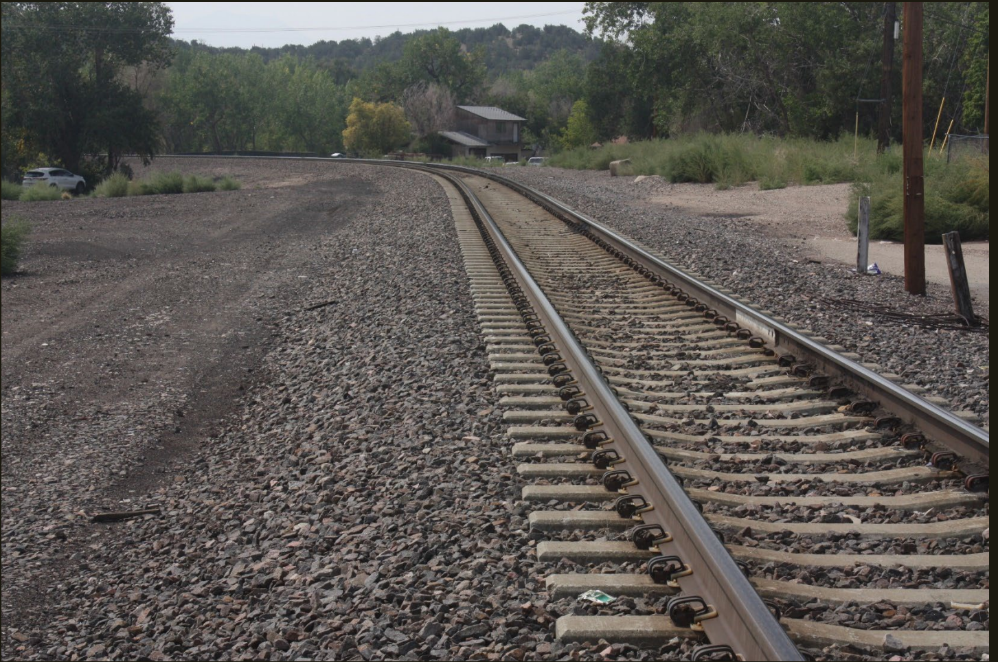
Southwestward view of the UPD&G (1895) at the same location as previous. The concrete ties continue to Trinidad.
