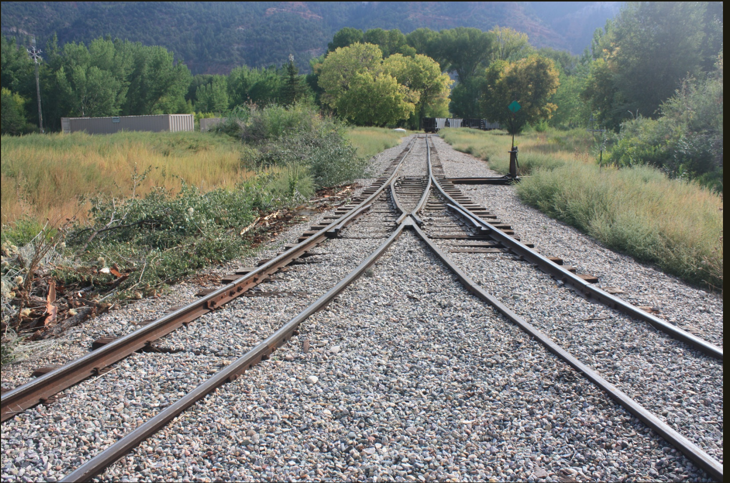
Eastward view of the tip of the D&SNGRR wye. Note the stored cars in the distance.
