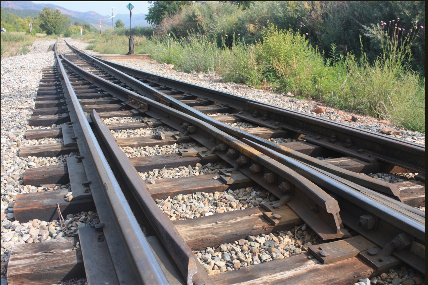
Now we are back at the D&RG Silverton Branch (1882n) looking north, toward Silverton, where the north branch of the D&SNGRR wye joins the historic narrow gauge railroad.
