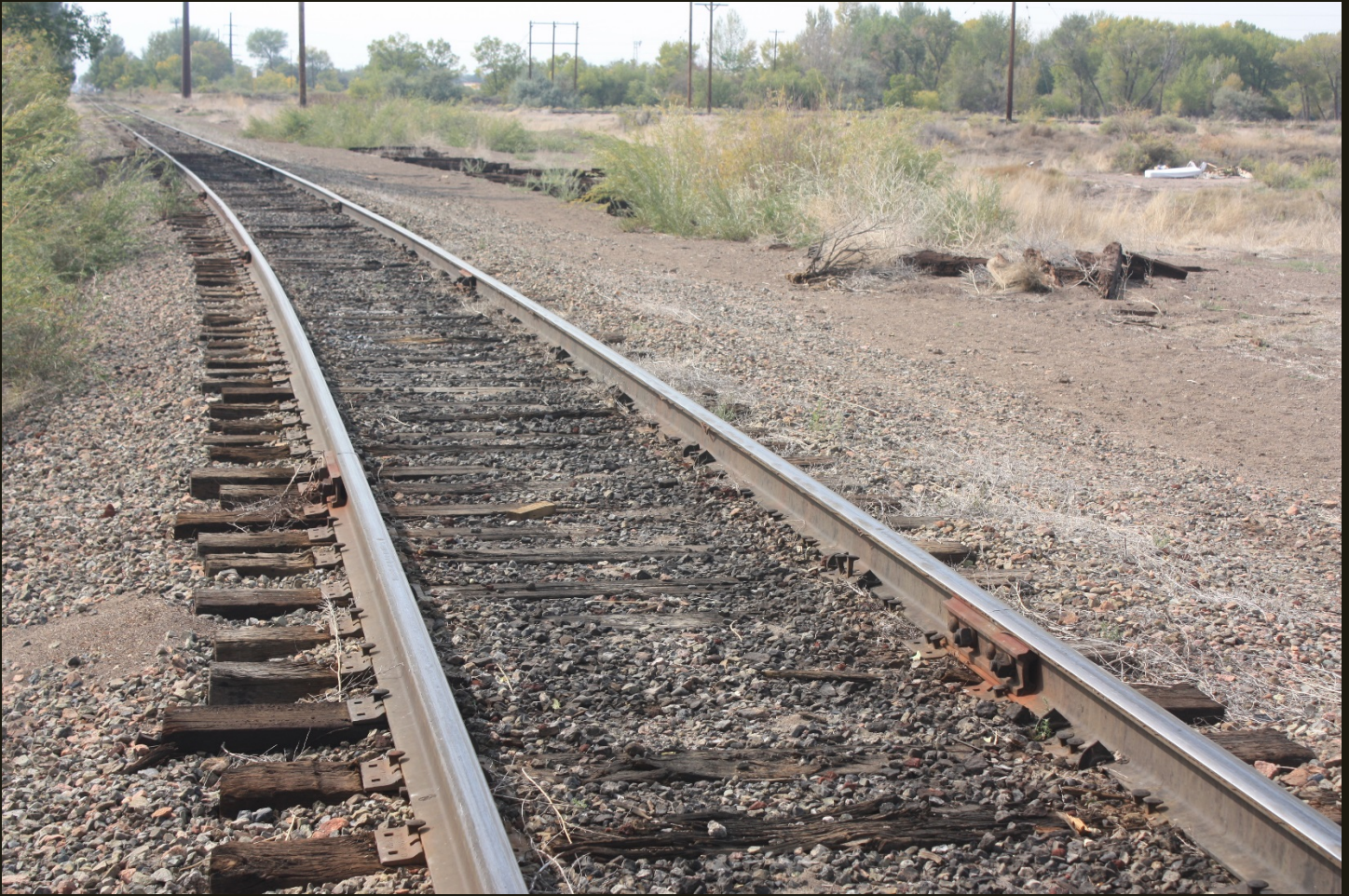
Now we are back at the D&RG San Juan Extension (1878n) looking west; the abandoned east branch of the wye is just out of sight to the right and the west branch track is visible across the entire photo in the distance. The line of loose ties on the ground to the right of the mainline track are the remains of a siding for the wye.
