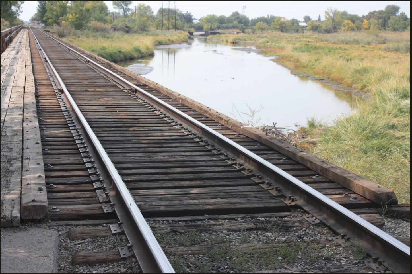
Westward view of the D&RG San Juan Extension (1878n) 100 feet west of the previous location. The bridge carries the mainline over the Rio Grande. The town of Alamosa is on the other side of the bridge.
