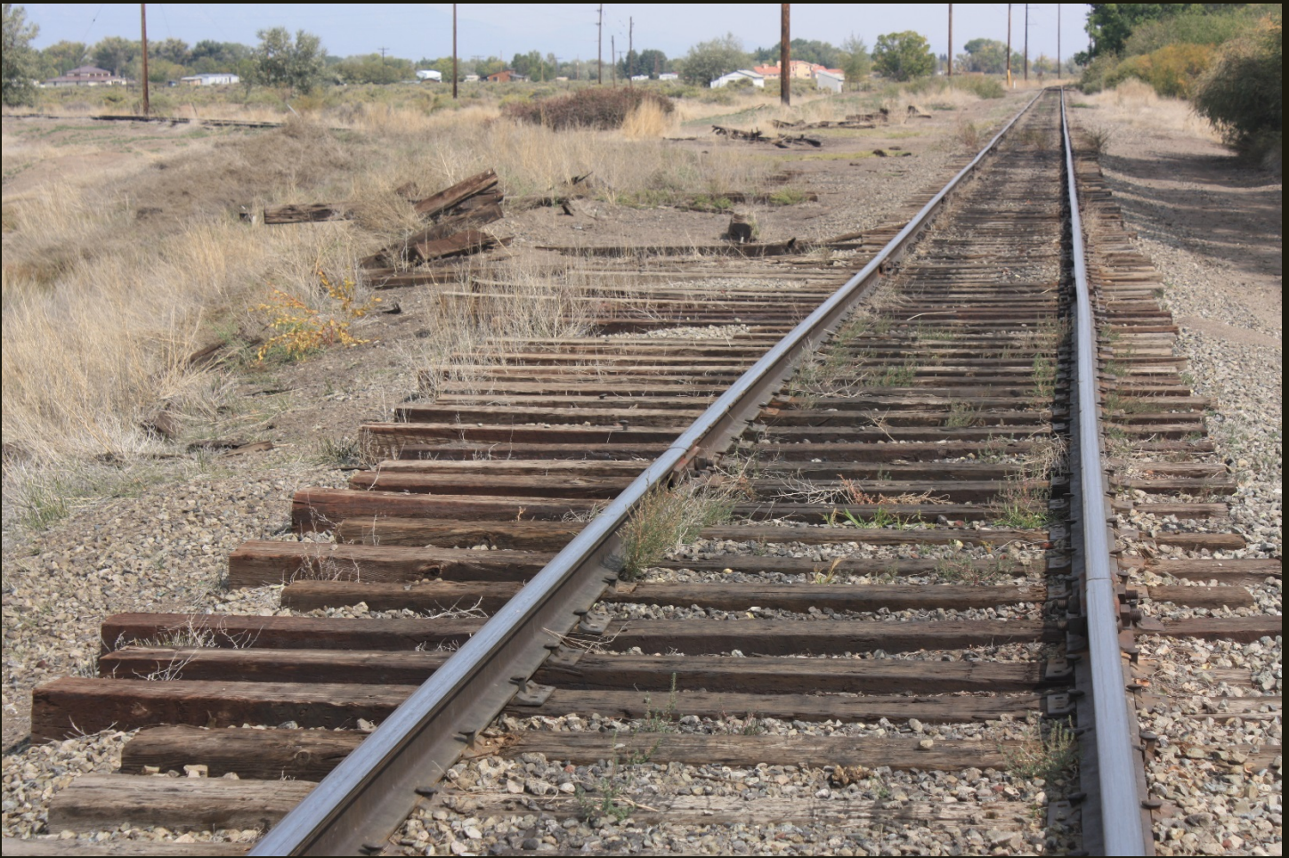
Eastward view of the D&RG San Juan Extension (1878n) 50 feet west of the previous location. The intact track in the foreground is the San Juan Extension mainline and the long ties extending to the left of the mainline rails were for the switch, now completely gone, for the siding for the wye for the Hooper Spur. The track for the west branch of the wye is visible in the left distance and the line of ties that represent the siding is in the middle distance, between the mainline and the utility poles.
