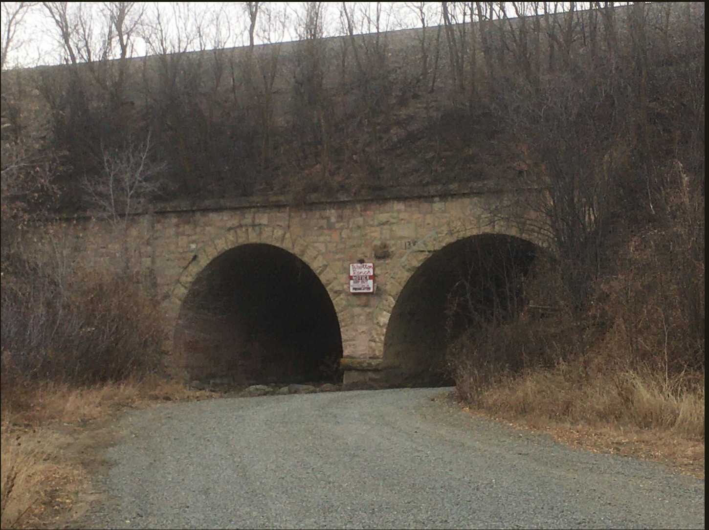
This is as close as I could get to the tracks north of the pass, where a ranch access road in Colorado crosses the tracks 2.25 rail miles north of the north entrance of the railroad tunnel. This tremendous fill grade and the beautiful stone tunnels through it give an idea of the construction feats on the approach to Raton Pass.
