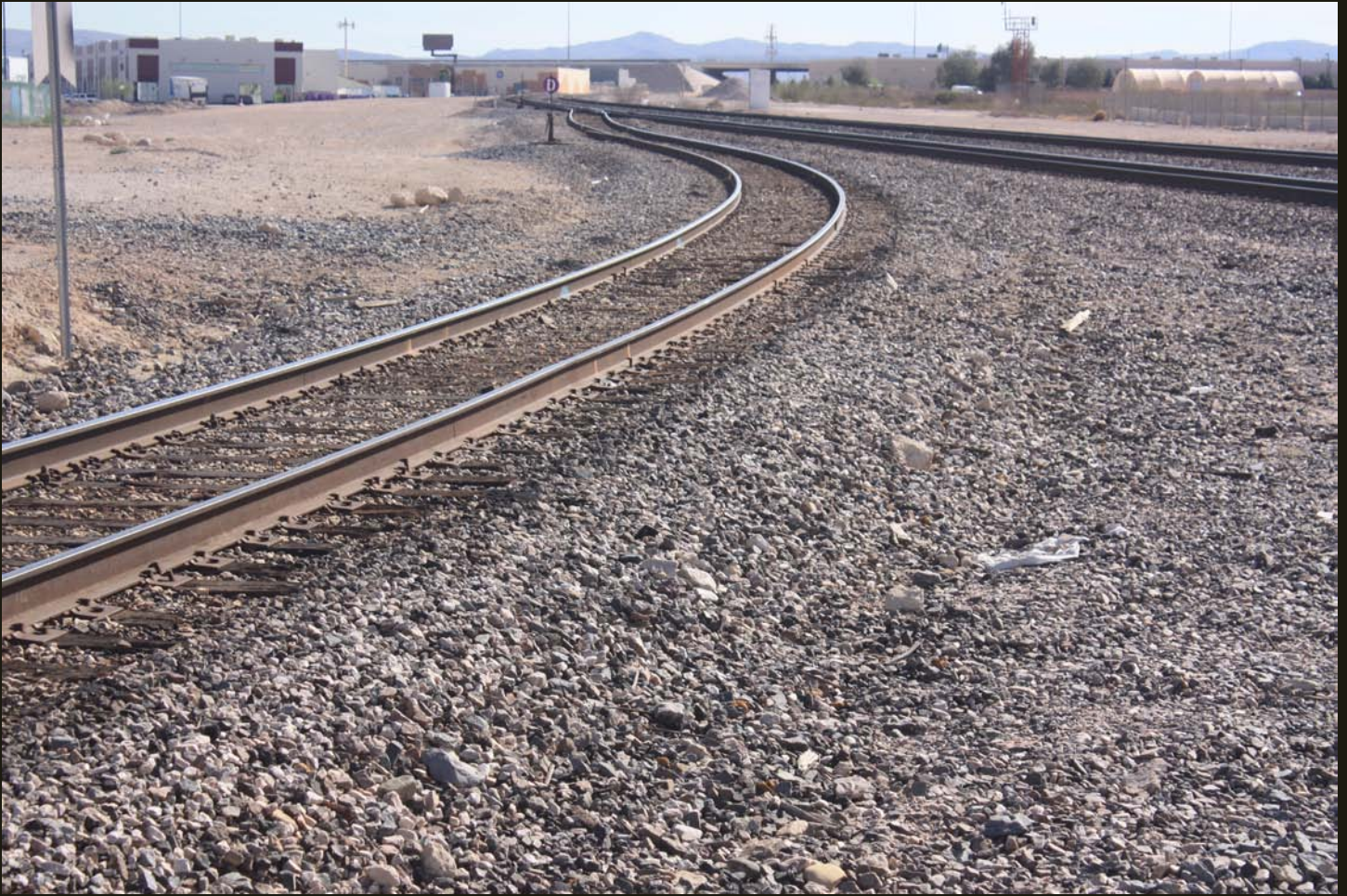
Another southwestward view of the south branch of the wye for the LA&SL Boulder City Branch (1931), with its connection with the SPLA&SL (later LA&SL and now UP) in the distance.
