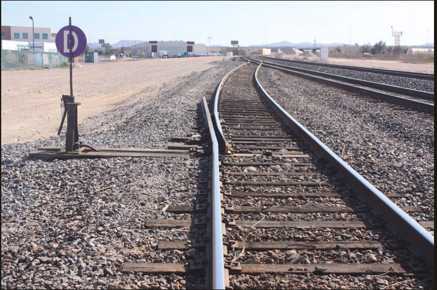
Southwestward view of the SPLA&SL a few steps east of previous location. The track in the foreground is the south branch of the wye for the LA&SL Boulder City Branch (1931).
