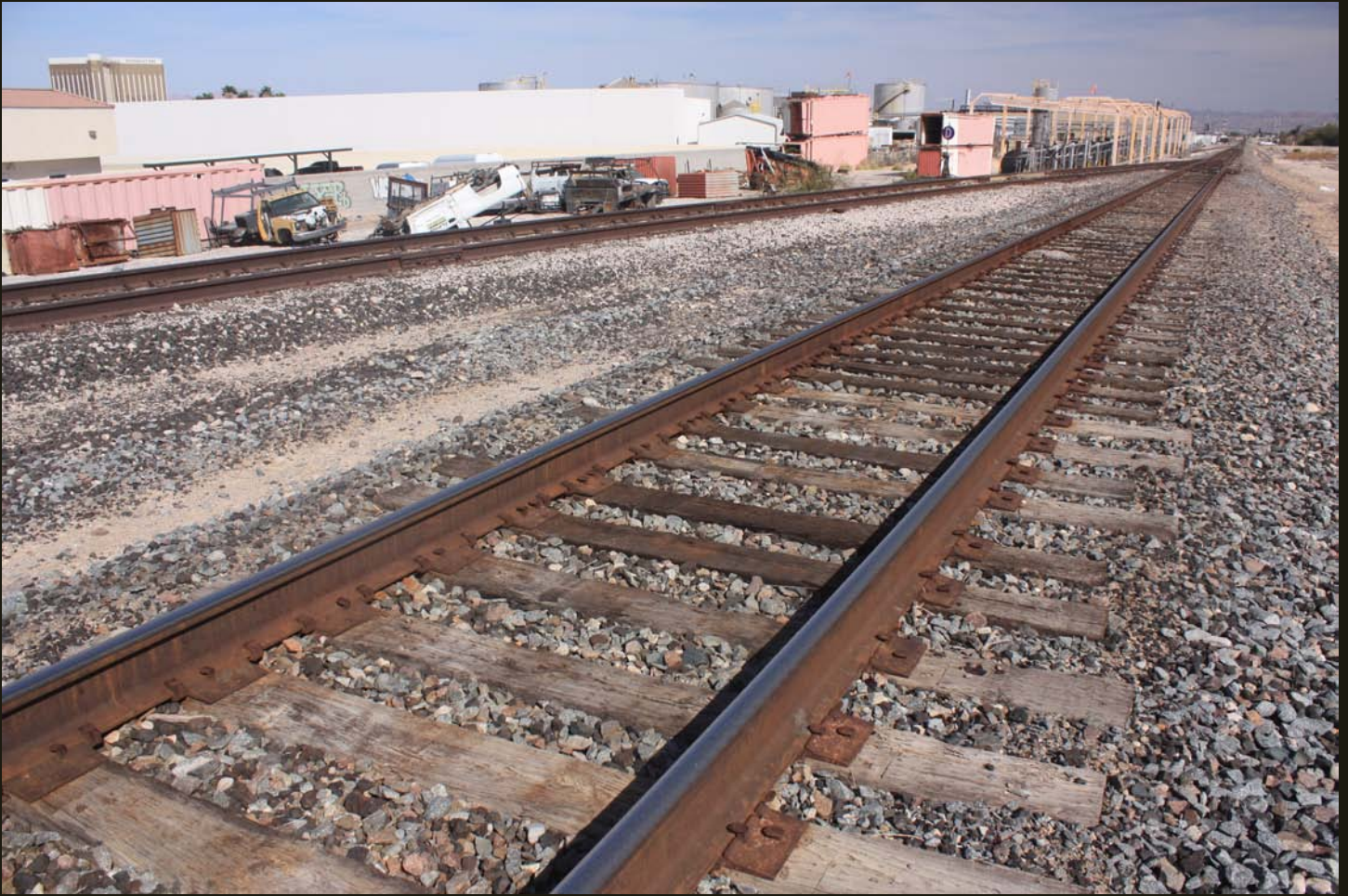
Eastward view of the two branches of the wye for the LA&SL Boulder City Branch (1931), same location as previous. The single track heads east to Boulder City in the right distance.
