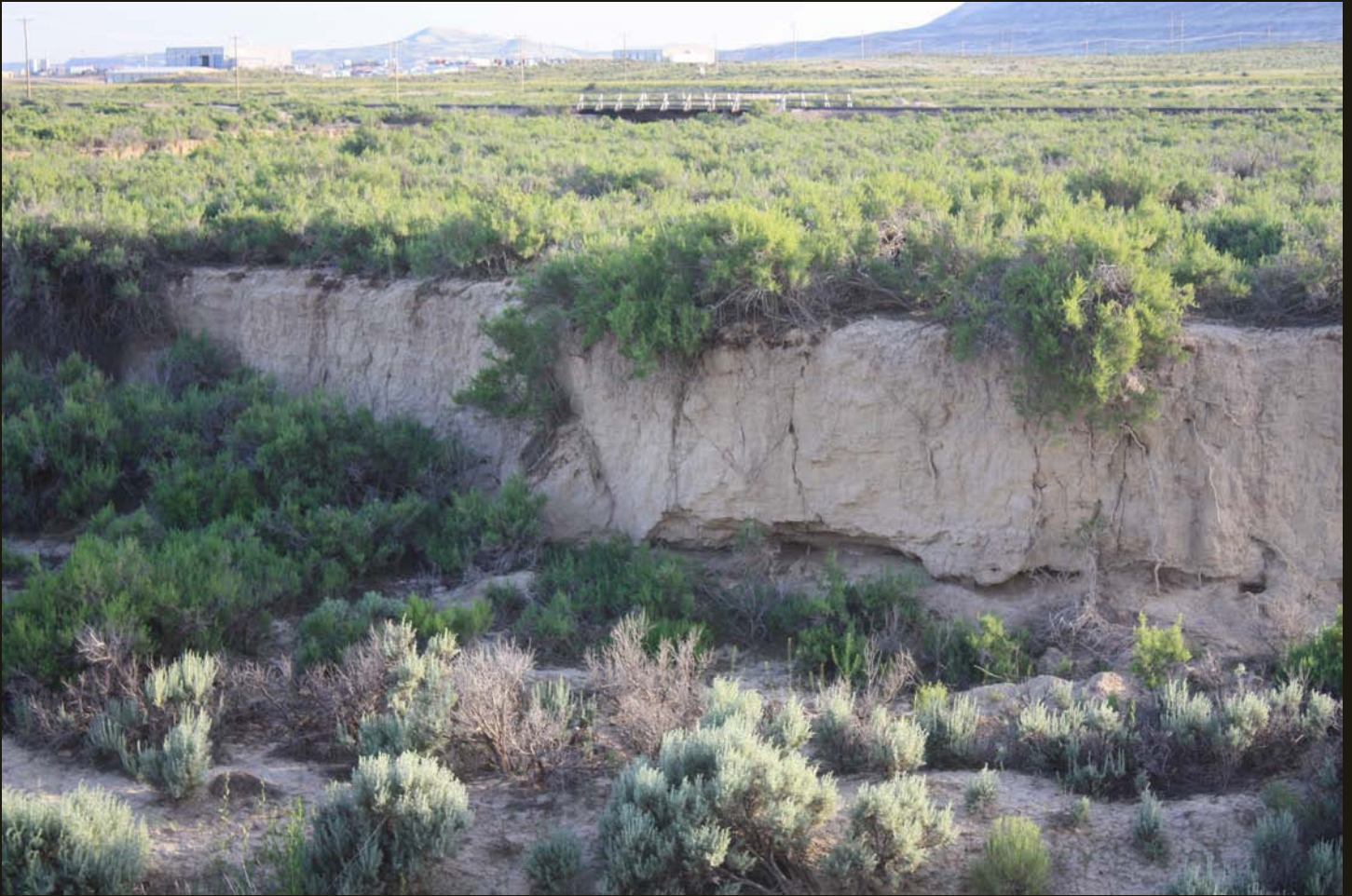
Westward view of a bridge that carries the Winton Branch over dry Killpecker Creek, about a quarter mile north of the Reliance Spur. The bank and dry bed of Killpecker Creek is visible in the foreground. The tracks end 500 feet to the right (north) of the bridge.
