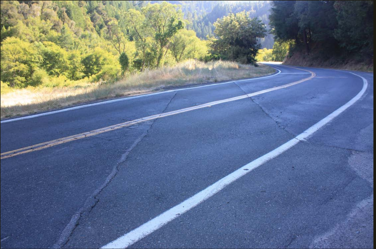
Railroad scar across California Highway 162; the tracks in the previous photos are in the grass across the street and behind the viewer.
