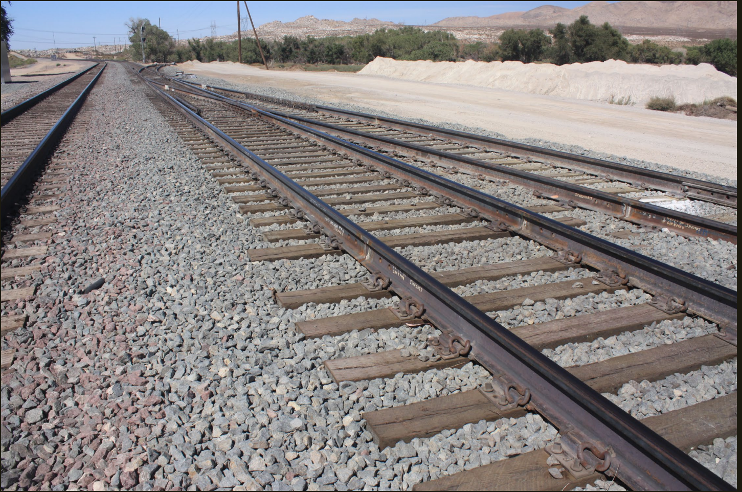
Northwestward view at the same location as previous, where the MN sidings have converged to one track, which joins one of the tracks of the CS/AT&SF/BNSF mainline in this view. The switch just beyond the MN switch goes to a 150-foot spur, probably a remnant of an abandoned siding.
