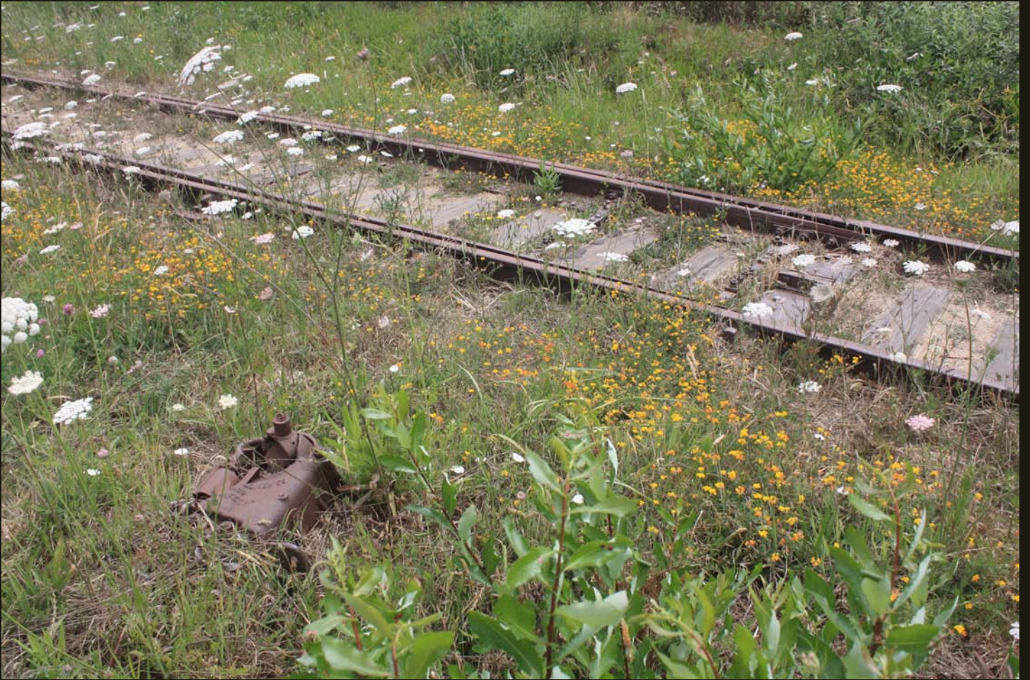
Another view of the same switch as previous, showing what's left of the rusting switch mechanism.
