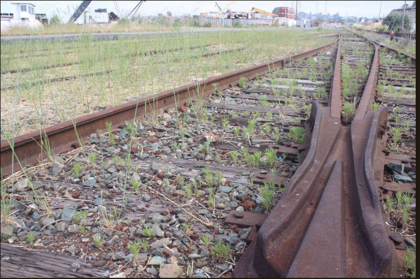
Close-up of a switch at the Vallejo yard.
