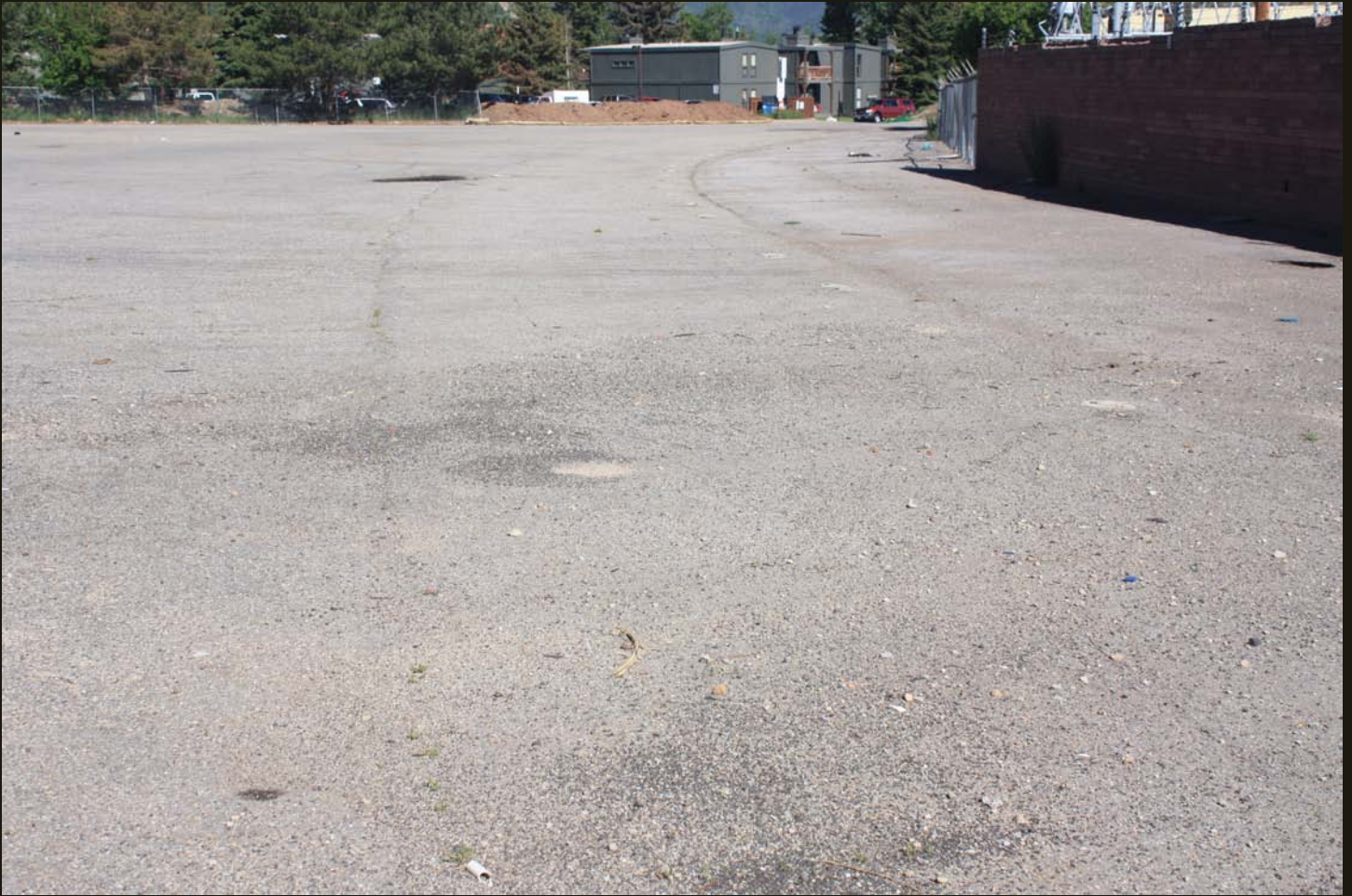
This parking lot behind commercial buildings in Park City is more interesting than it appears; it is the wye for turning E-PC engines at the end-of-the-line at Park City. The curved cracks in the asphalt are a patch over the original curved track of the wye, in this view facing away from the end of the mainline behind the observer. The other branch of the wye runs along the far side of the asphalt area, which is similarly curved.
