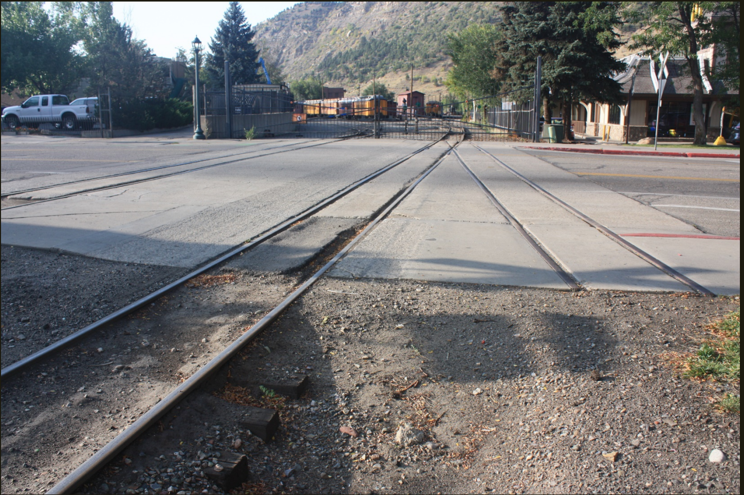
Southward view at the same location as previous, showing the mainline on the far left, the first branch off the mainline going into the D&SNGRR railyard in the middle, and an abandoned spur on the right. An 1898 topo map shows that the mainline is on the original D&RG Silverton Branch (1882n) alignment, including the curve to the left (east) on the other side of West College Drive. The topo map does not show either of the two spurs visible here.
