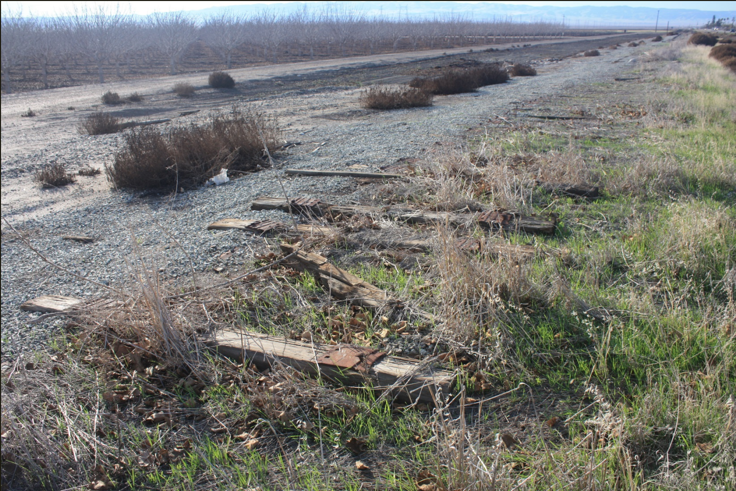
Southwestward view of the MS (1893), 2,000 feet west of previous location. The track is gone, some ties are still in present.
