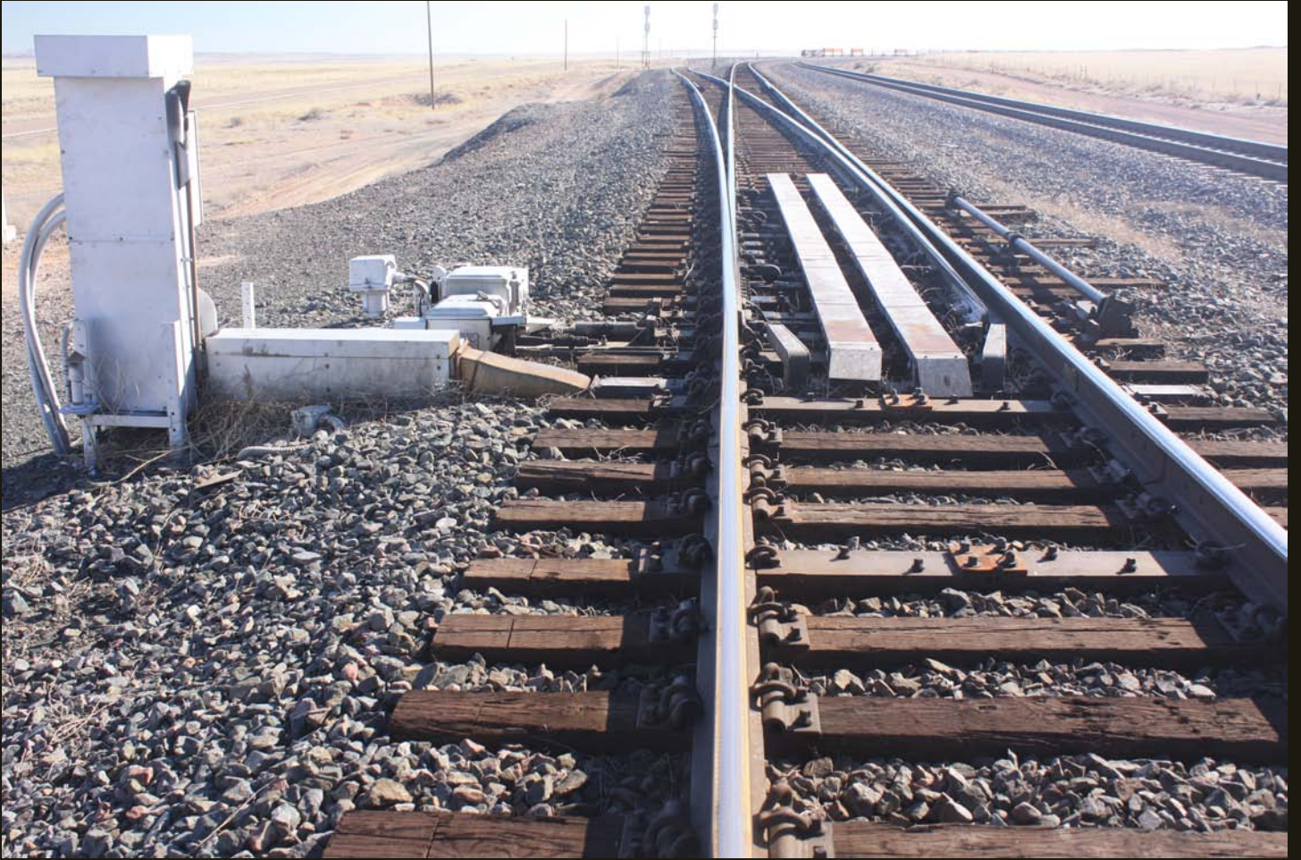
Modern switch for the siding at Culebra.
