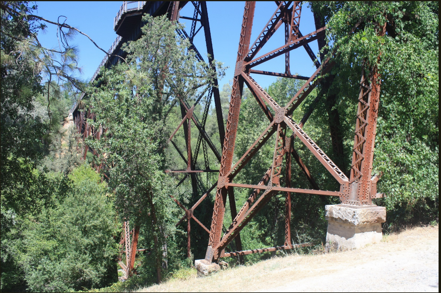
Northward view of the S&P (1888), 3,000 feet northeast of the previous location where the alignment crosses Weber Creek. The original 1888 trestle was constructed of wood and the SP replaced it in 1903 with the current metal structure. The tracks are gone but the trestle now carries the El Dorado Trail over the creek.
