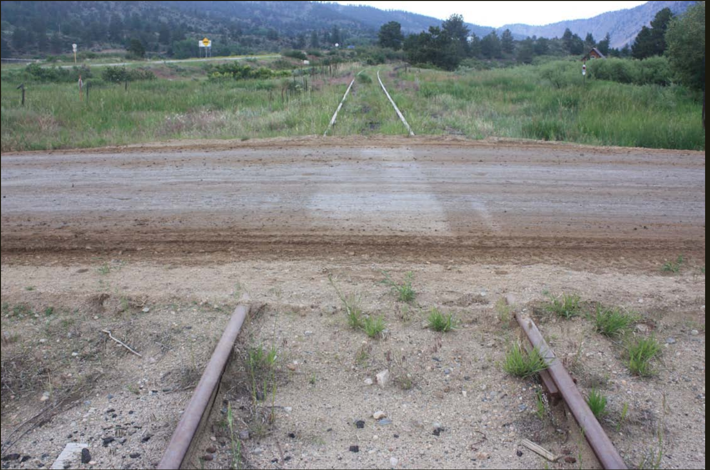
Three miles south of the previous photo, the inactive D&RG line is buried; the D&RG Tennessee Pass Route is on its way to abandonment.
