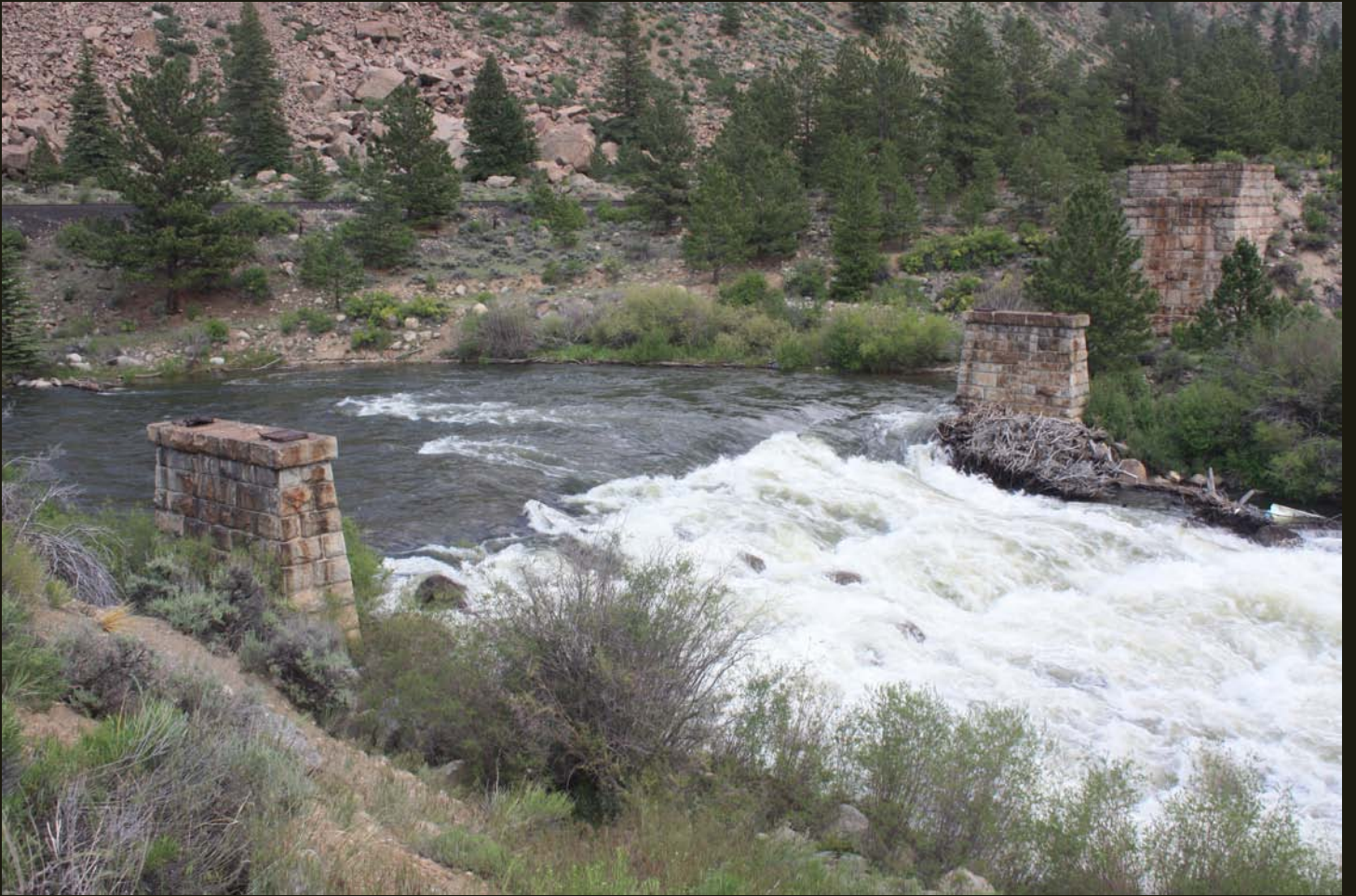
Another view of the CM bridge across the Arkansas River.; the D&RG (now inactive UP) tracks are on the far bank.
