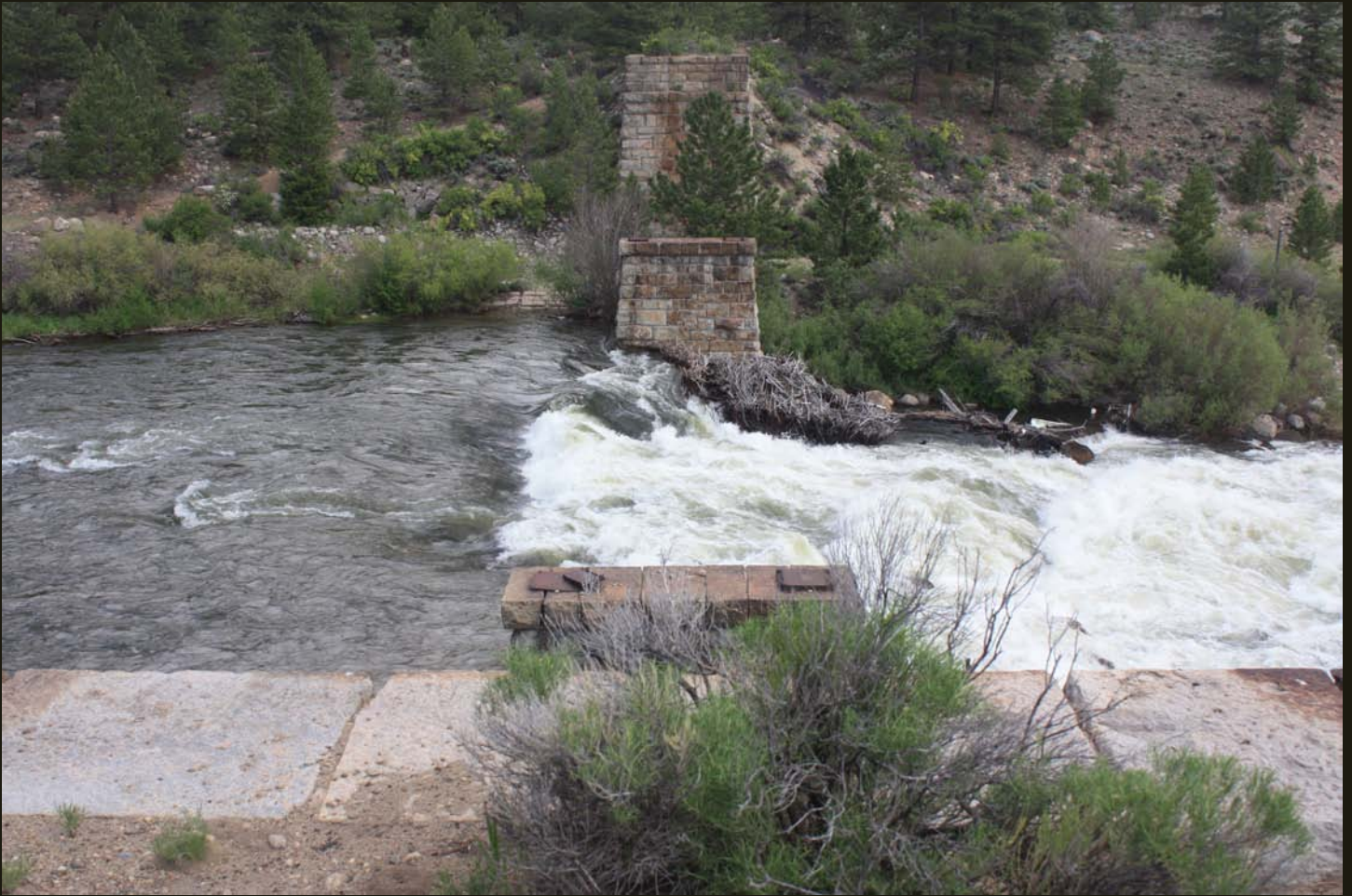
All four supports for the CM bridge across the Arkansas River near Clear Creek Reservoir. The CM was scrapped in the early 1920's, so these foundations have stood for nearly a century since the rails were removed.
