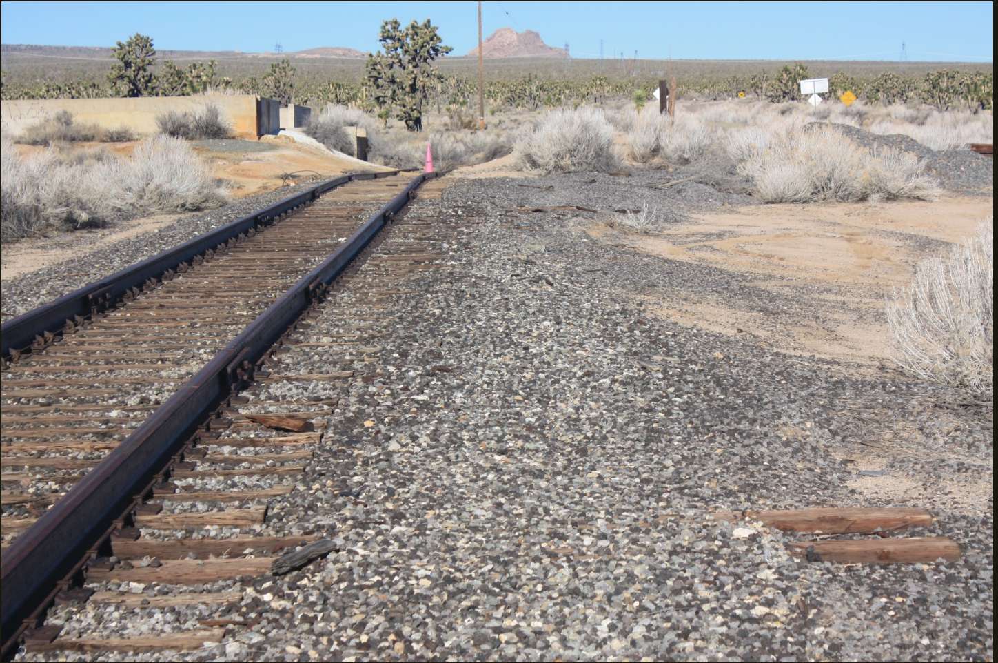
Northwestward view of the straight track just past the tip of the Cima wye. The same concrete foundation is to the left of the track and the same gray ballast gravel is to the right of the track. Note the two long ties in the foreground, indicative of a former switch lever at this location. Beyond the switch lever ties, the track ties become progressively longer in the distance. These ties were beneath the track that curved to the right past the switch lever. Thus, the track that once extended north-northeast 2,000 feet from this location was connected to the wye via a switch, which is completely removed except for the ties.
