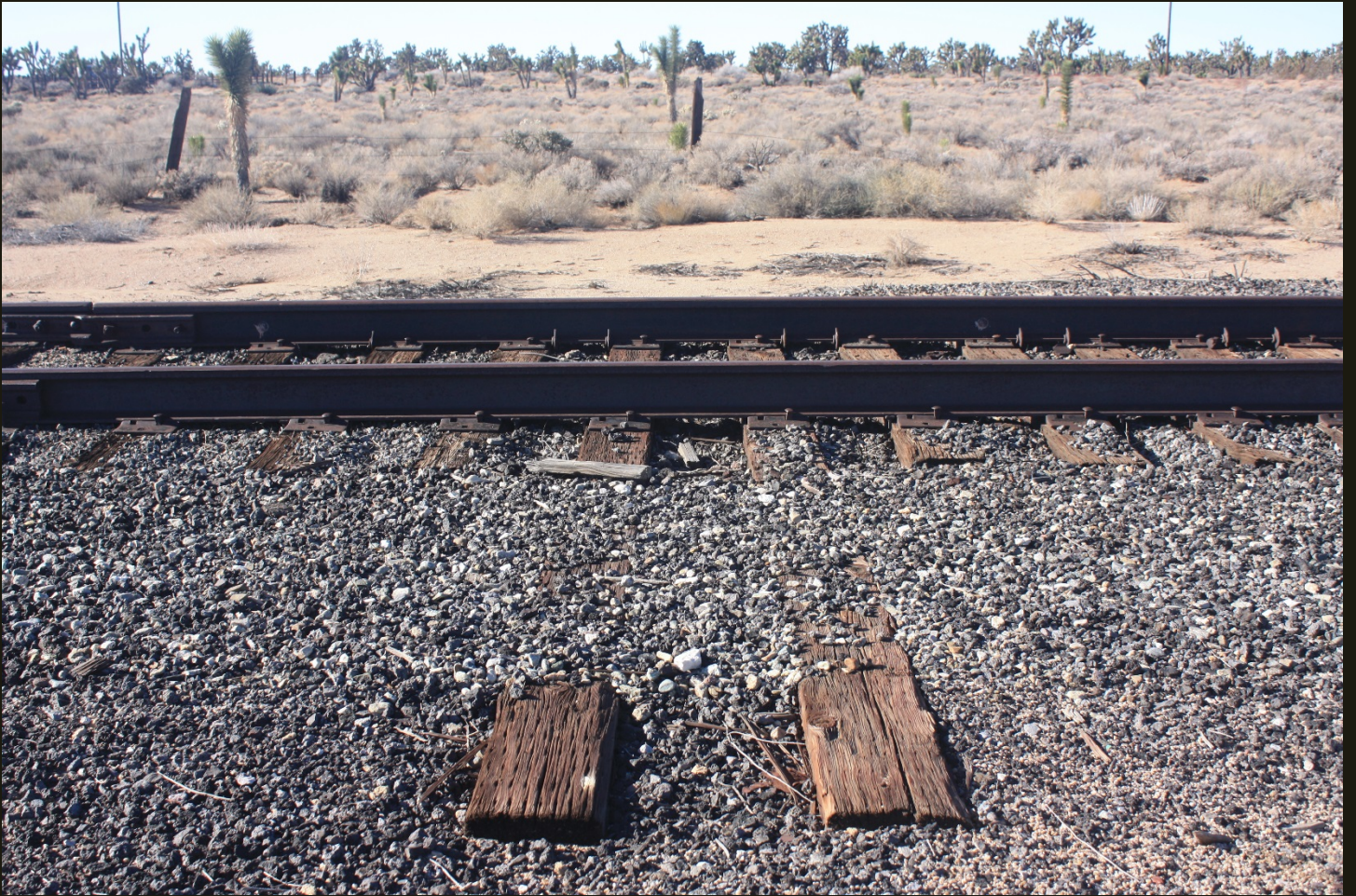
Southwestward view of the two long ties for the former switch lever.
