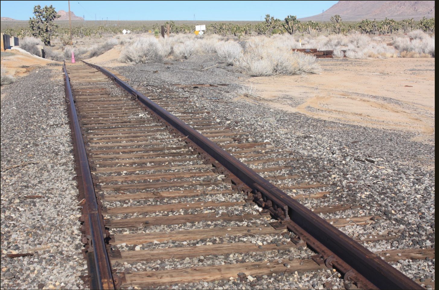
Slightly closer view of the progressively longer ties for the former switch. Note also the gray gravel, in this view more clearly curving to the right.
