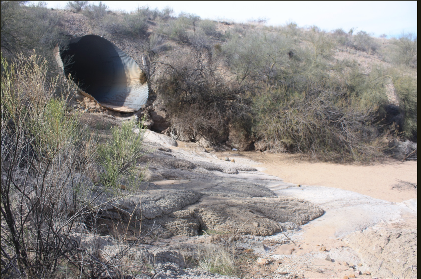
Culvert under the fill grade for the SMA (1955) switchback to the San Manuel copper mine, a few steps south of previous location.
