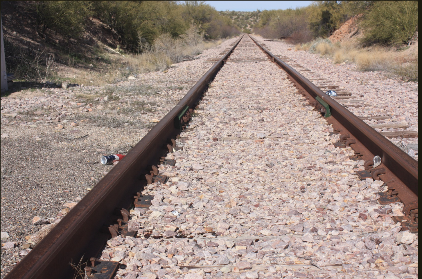
Northwestward view of the SMA (1955), 2,000 feet south of the previous location. The trestle is just around the distant bend.
