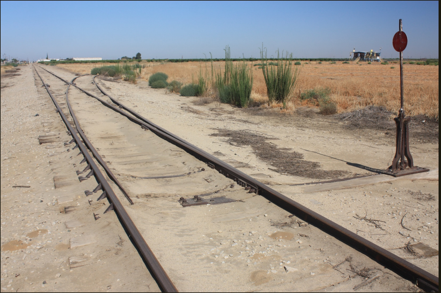
Westward view of the SP Arvin Branch (1923), a quarter mile east of the previous location. The curved track to the right (north) is the east branch of a wye that leads 1,500 feet to a petroleum storage facility. The west branch of the wye splits from the mainline where the orchard starts to the right of the track in the left distance.
