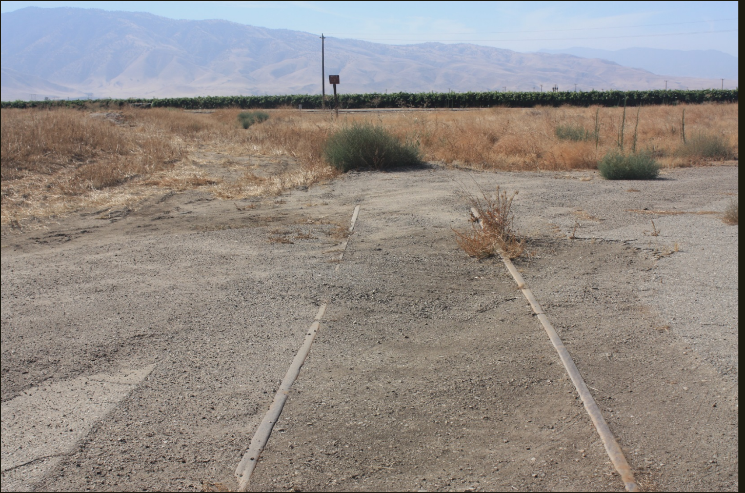
Southward view of the east branch of the wye, 500 feet northwest of the previous location. The track is obviously not being used.
