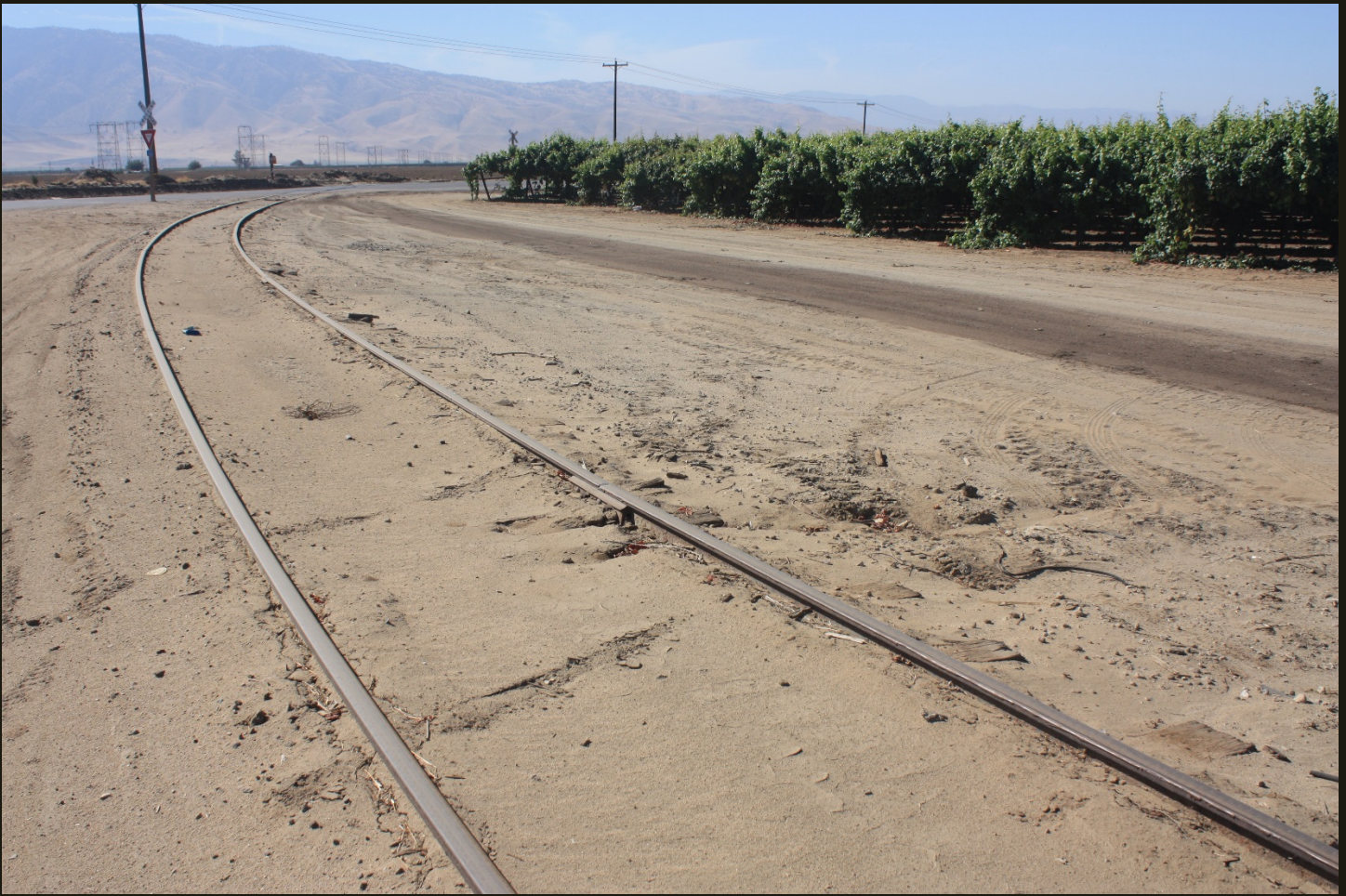
Southeastward view of the SP Arvin Branch (1923), same location as previous, where the alignment makes its second and final 90-degree curve to head due south to Arvin. In the distance, the tracks cross north-south-running Tejon Highway.
