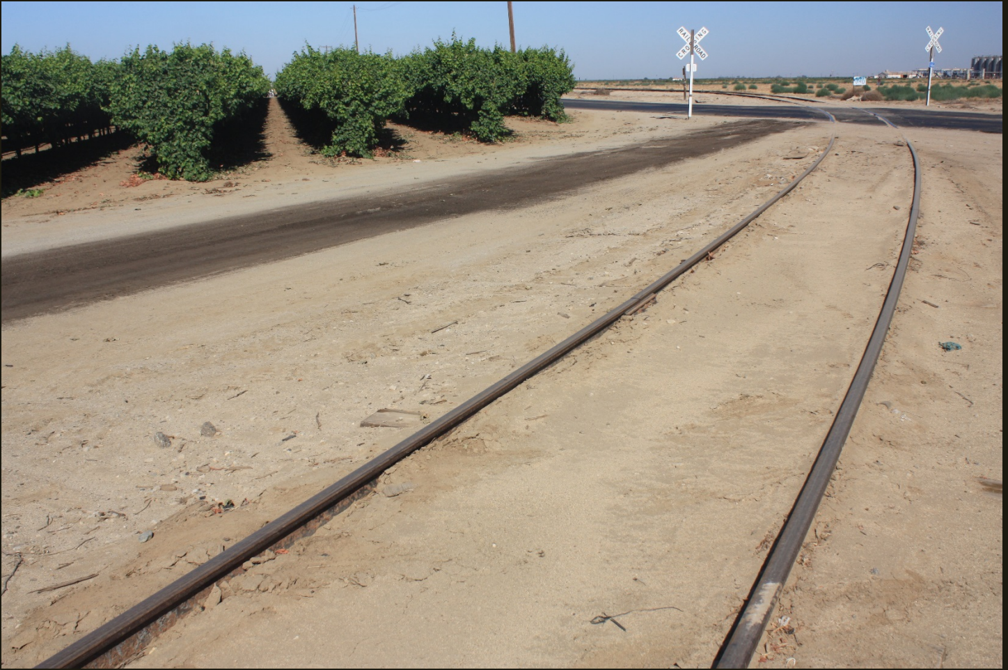
Northwestward view of the SP Arvin Branch (1923), 900 feet east of the previous location, where the alignment makes its second and final 90-degree curve to head due south to Arvin. The tracks cross east-west-running DiGorgio Road.
