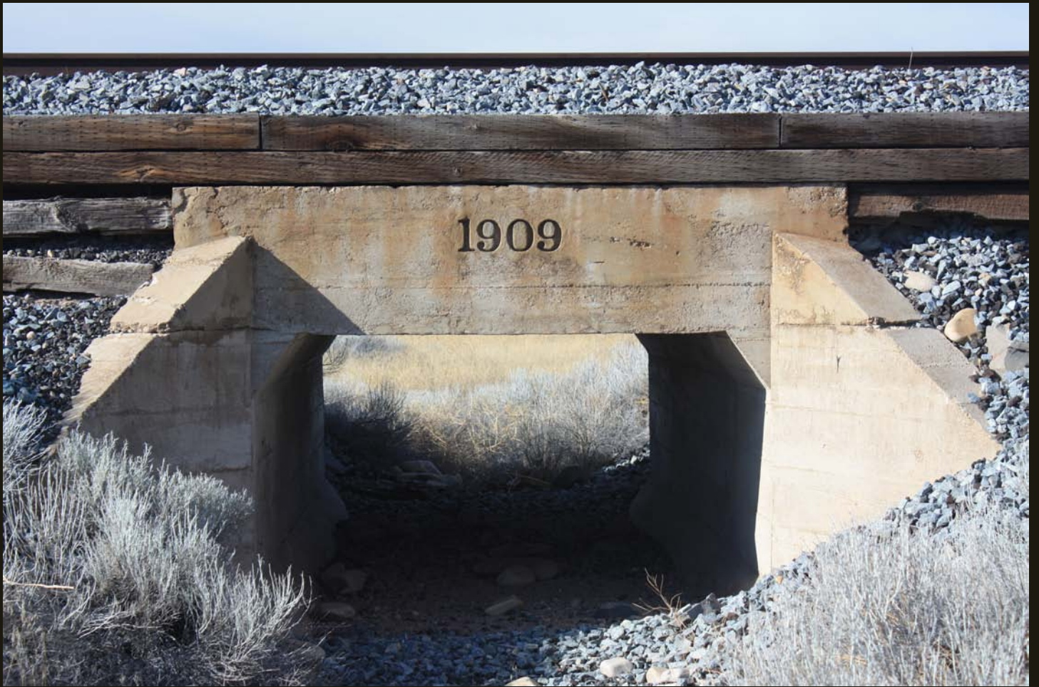
Although the SPLA&SL mainline was completed in 1905, this culvert on the mainline at Lund was apparently constructed or upgraded in 1909.
