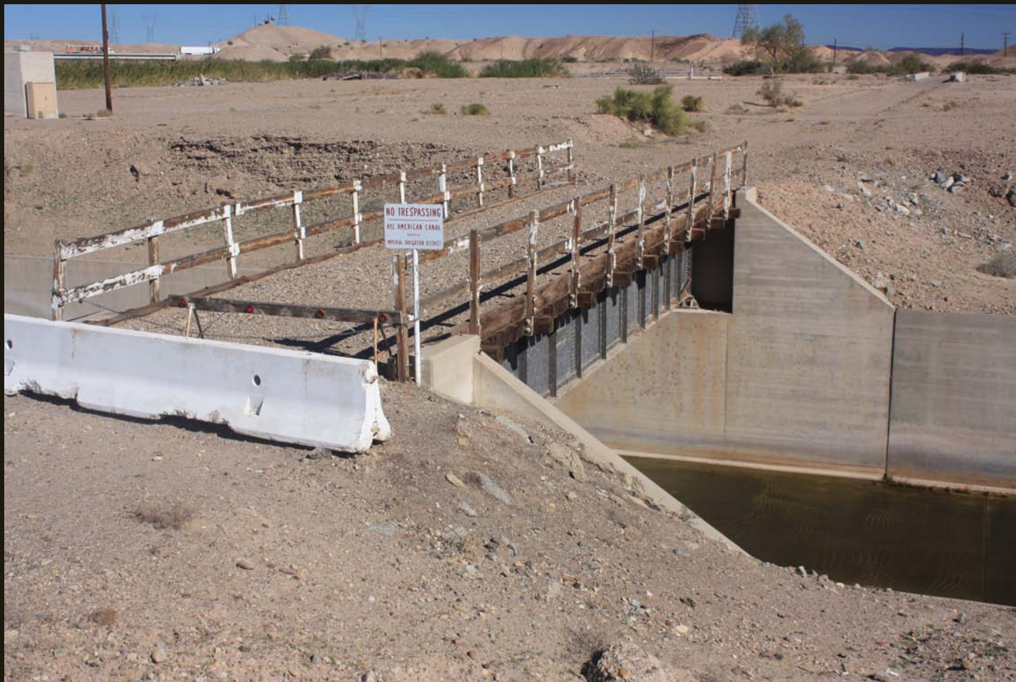
One mile south of Araz Junction, where a bridge carries the SP Inter-Cal (1904) over a control channel for the All American Canal. The overgrown reeds to the left (northwest) is the canal and the Colorado River is to the right (out of sight to the southeast) in this northward view. A second bridge in the right distance carries the grade over another control channel.
