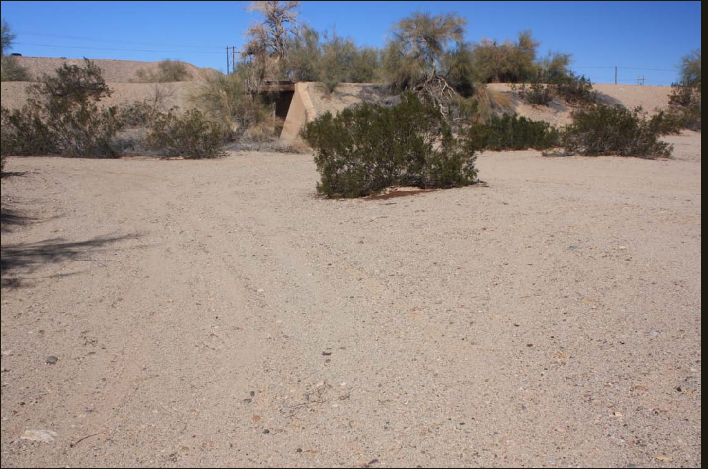
Northward view of the same fill grade and small bridge as in the previous photo.
