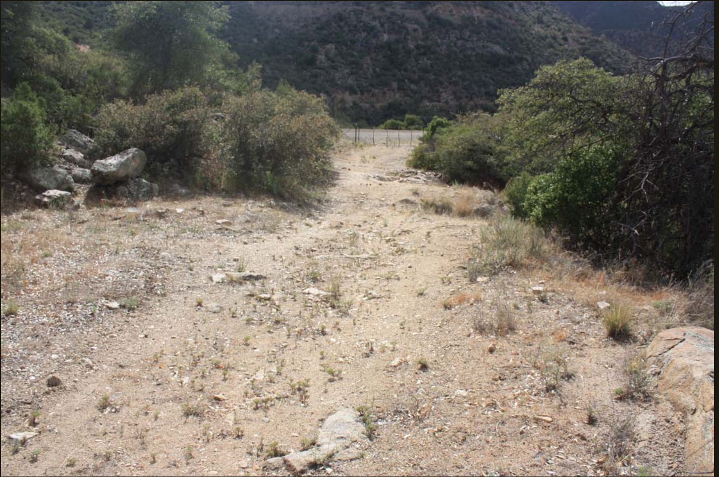
Another view of a switchback. The grade in the foreground was for a switch and single track and the re-graded automobile U-turn is in the distance.
