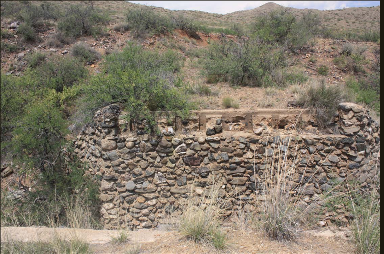
Another view of the old BM(?) bridge abutment. Note the cut grade beyond the abutment.
