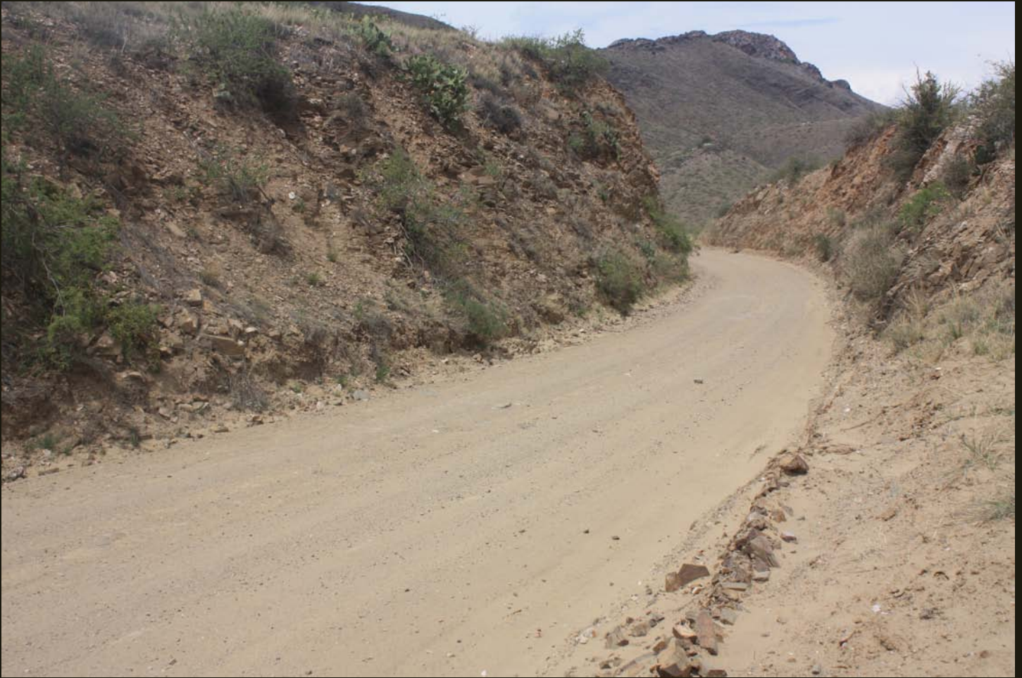
Cut grade on the BM on the climb up to Crown King.
