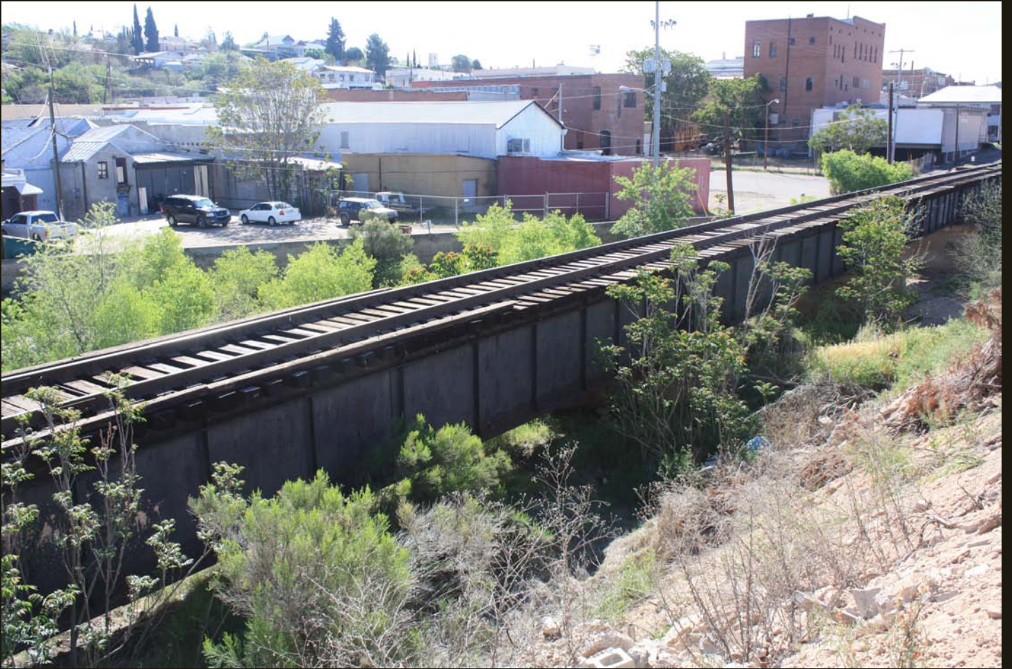
The beginning of the AE Miami Extension on the west side of Globe required a substantial bridge.
