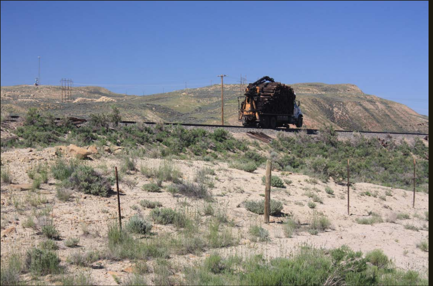
A specially built rail truck picks up discarded ties along the UP mainline near Point of Rocks.
