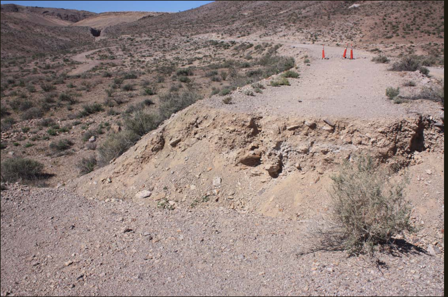
Westward view of the LV&T (1907) 2.5 miles west of Beatty, where a fill grade is washed out and a deep cut is present in the distance.
