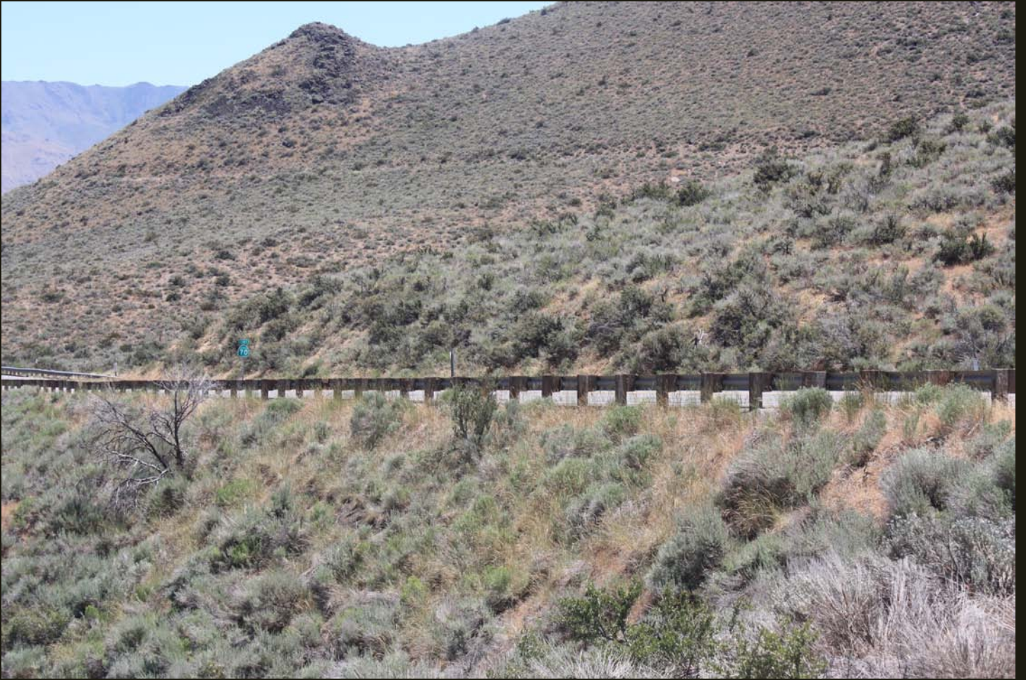
Southeastward view of the SV (1896n) cut grade on the hillside, with California Highway 70 below it, just east of Beckwourth Pass.
