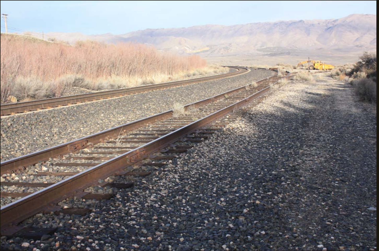
Eastward view of the WP mainline and siding at its connection to the WP Reno Branch. Petersen Mountain is in the background. Note the bundle of ties laid on the siding (right-hand track) just beyond the switch.
