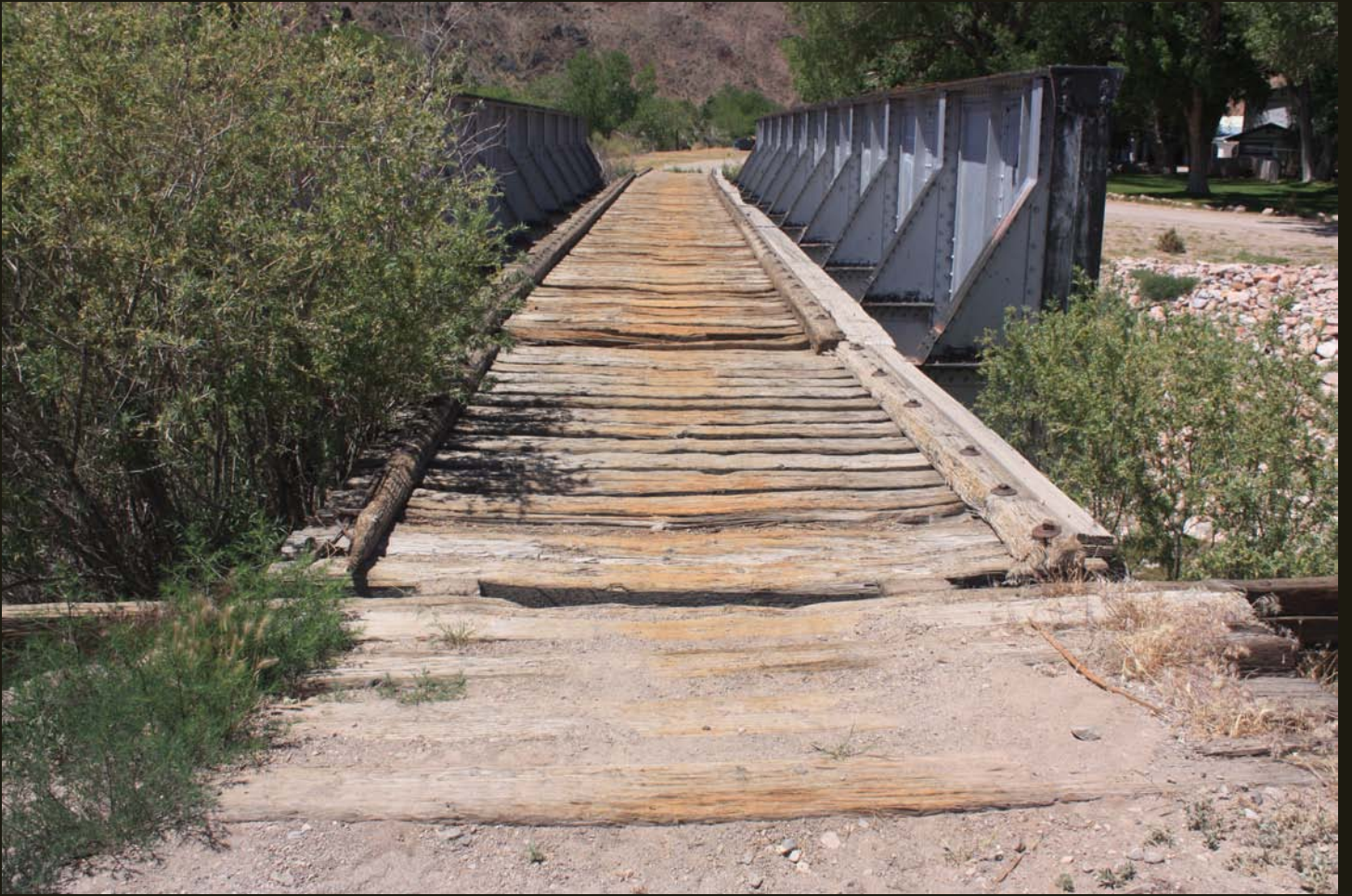
Northwestward view of the C&P (1907) bridge over Clover Creek, 400 feet northwest of the end of track.
