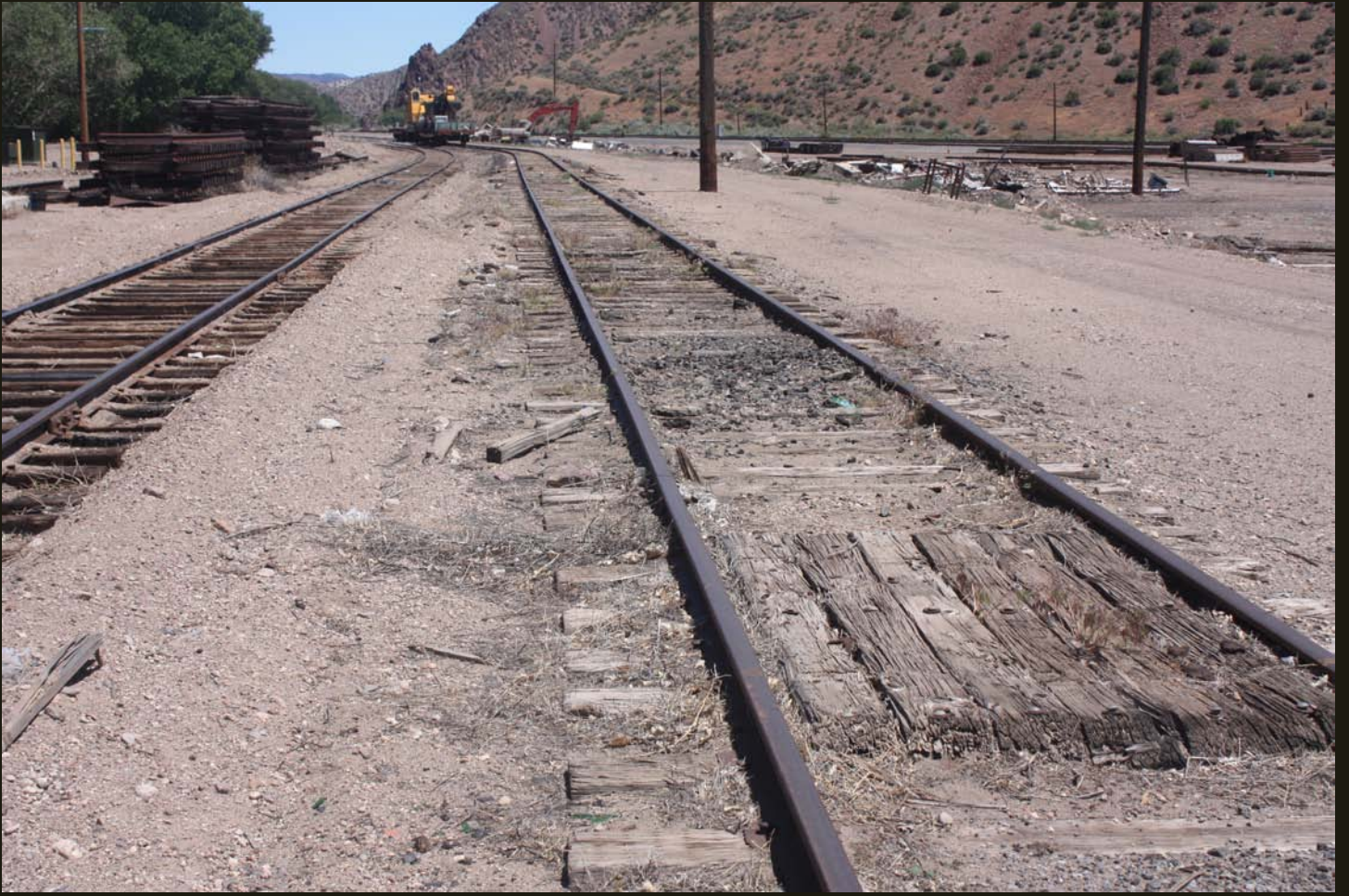
Southeastward view of the C&P (1907), showing its curve toward the north and Pioche.
