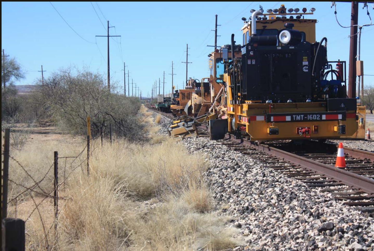
Westward view of the Pima Spur, just west of the previous location. Note the stored maintenance vehicles and the tailings pile for the Pima Mine in the left distance.
