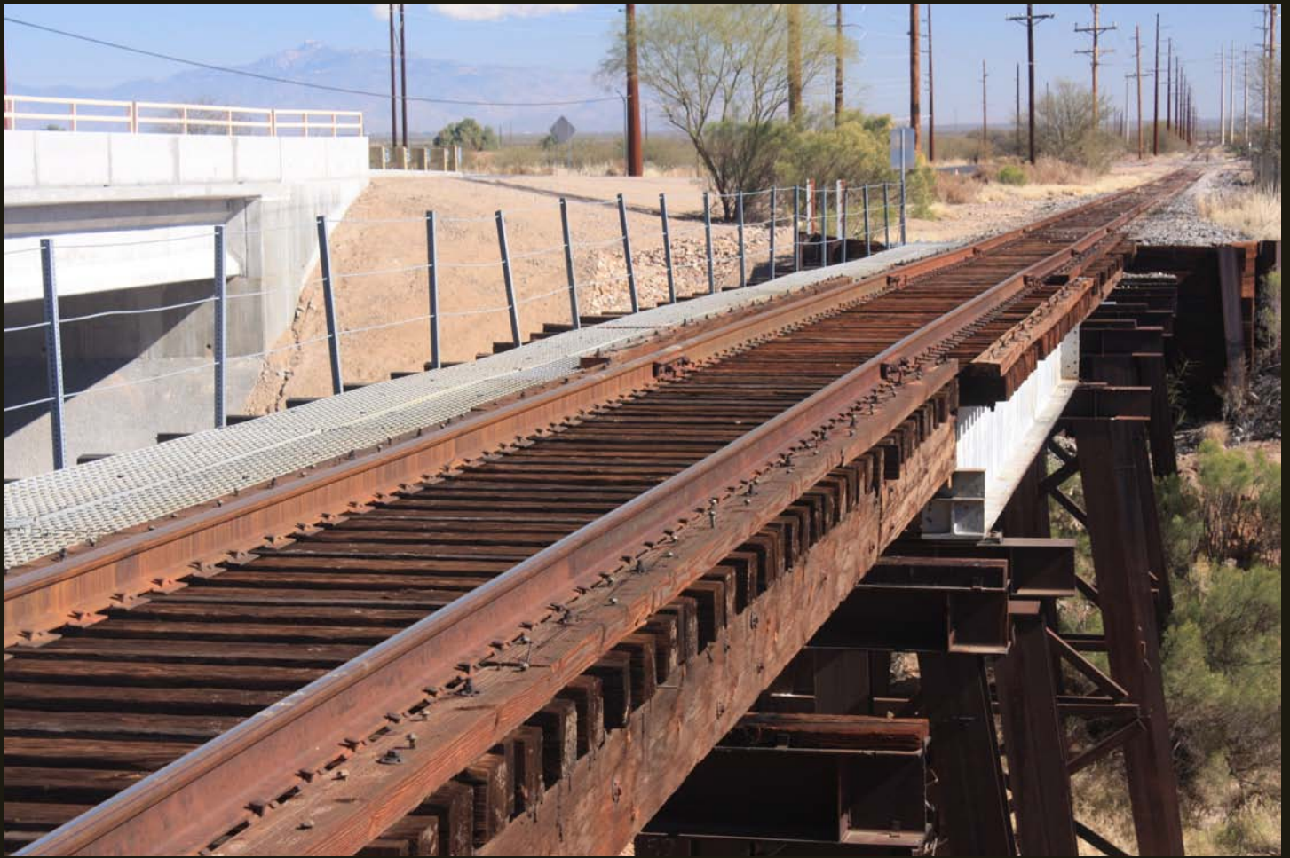
Eastward view of the Pima Spur, 1 mile west of the previous location, where a trestle carries the line over the currently dry Santa Cruz River.
