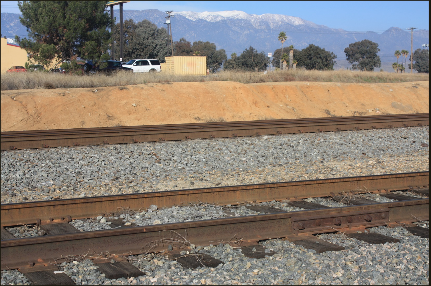
Northward view of the mainline double track and the bolted siding, with 11,503-foot Mount San Gorgonio in the distance. Note the slight cut to level the topography that slopes gently up toward Mount San Gorgonio.
