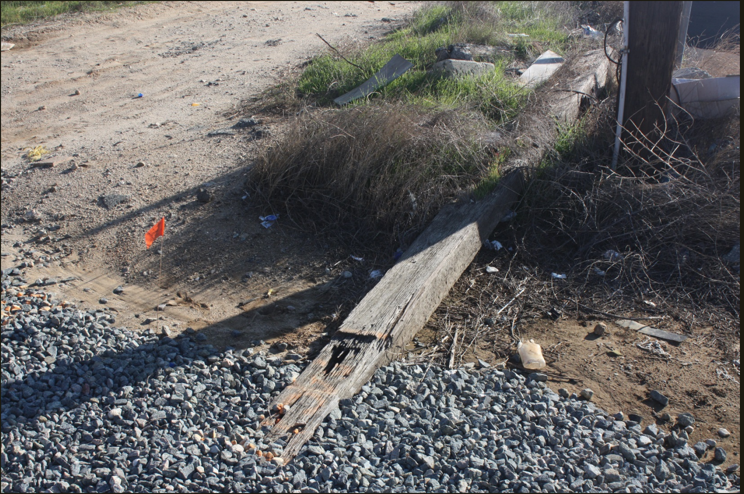
Closer view of the discarded tie. The tie is 12 feet long, much longer than a normal tie, with an indentation on the near end much wider than would be made by a simple rail plate. This was almost certainly one of two long ties used to connect a switch lever to a track switch. It could have been a switch for an old siding because the 1942 topo map shows three now-removed sidings that start 100 yards west of here. However, the proximity of the tie to the former wye makes the wye interpretation more likely.
