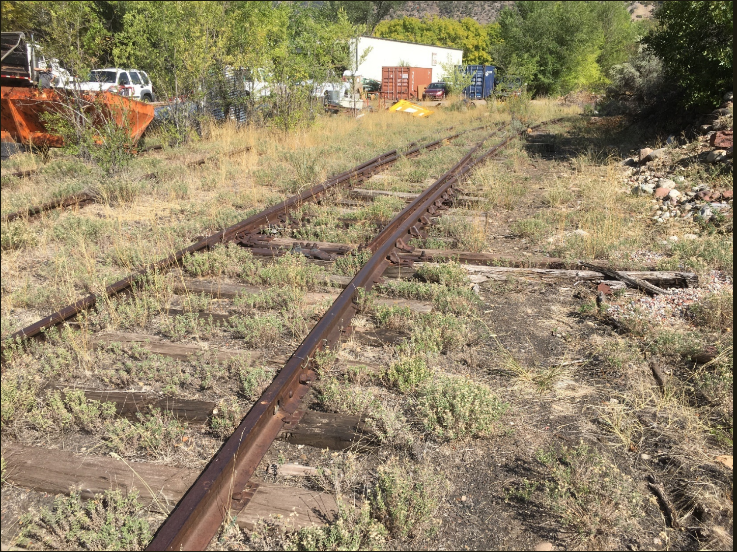
Northward view 100 feet south of the previous location. The track in the foreground is the east branch of the wye where it converges to a single track (the same switch as in the previous photo). The overgrown track on the left is the west branch of the wye.
