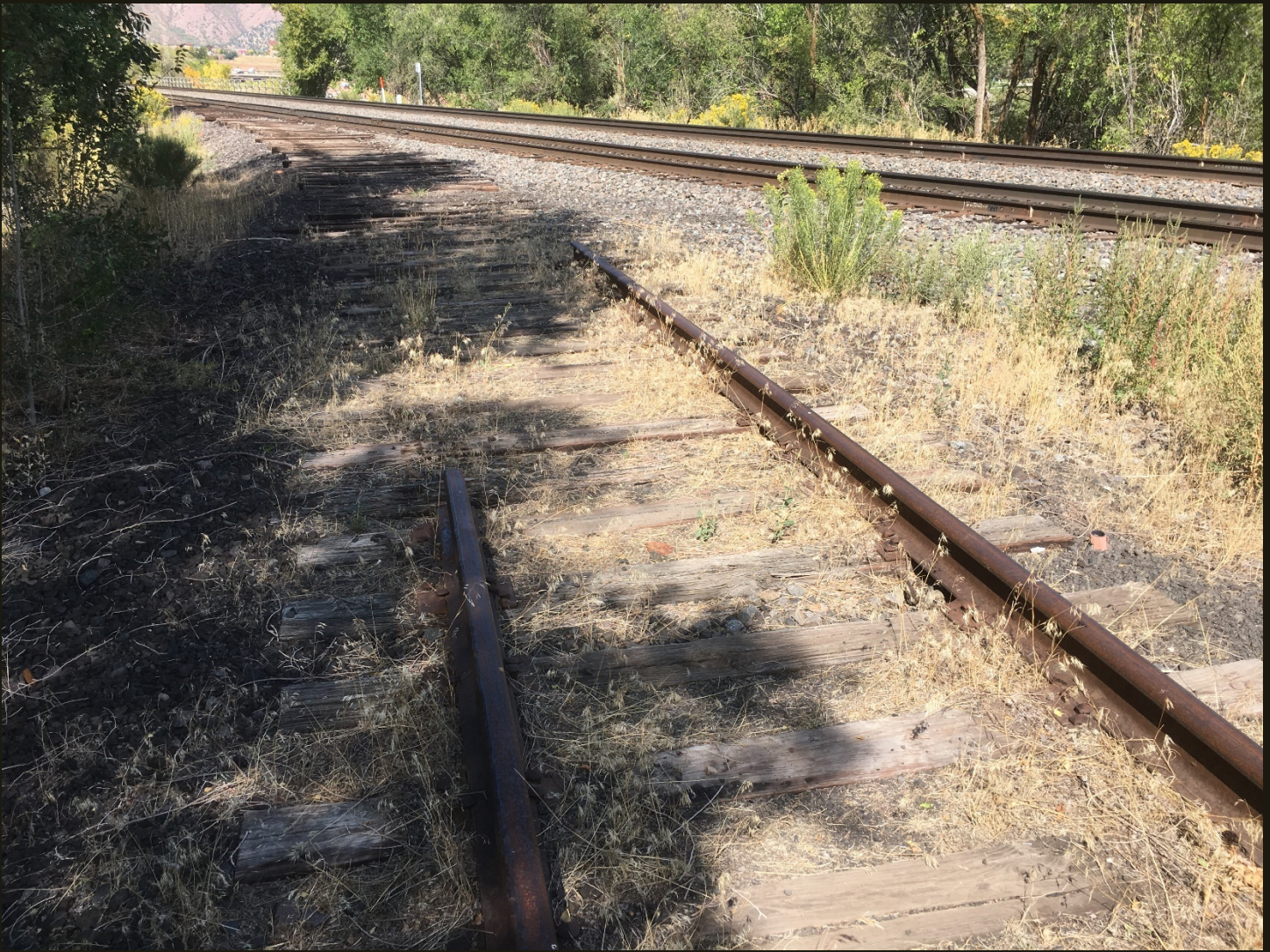
Northwestward view of the west branch of the wye 150 feet northwest of the previous location. All the ties are still present but the rails have been removed from the switch to the 1967 mainline.
