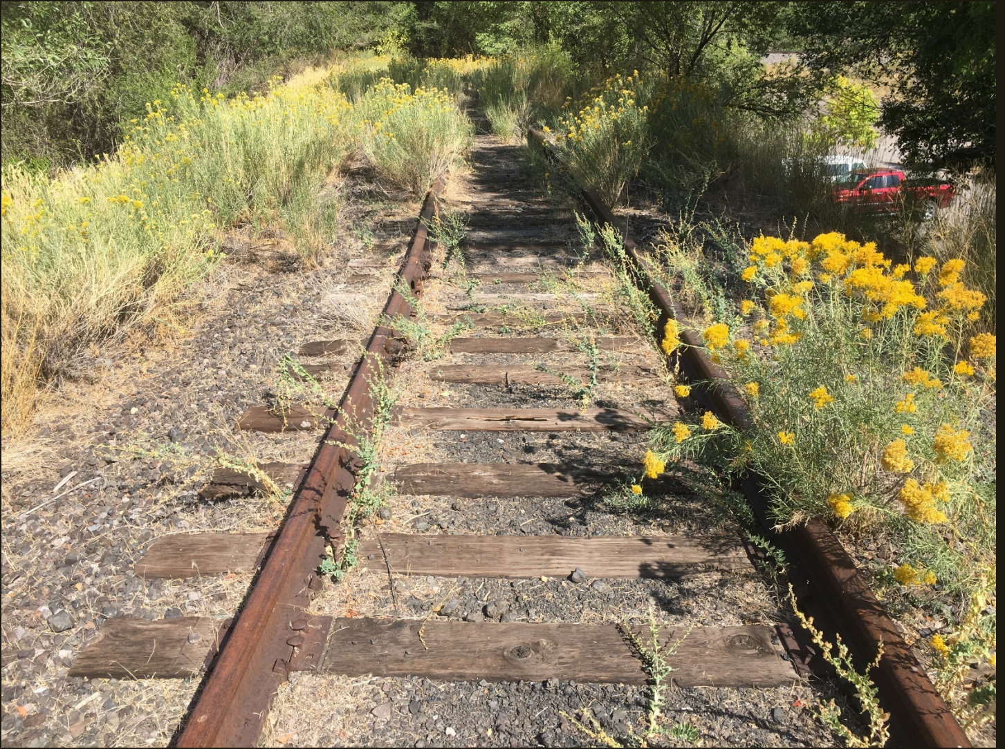
Northward view of the west branch of the wye 100 feet north of the previous location.
