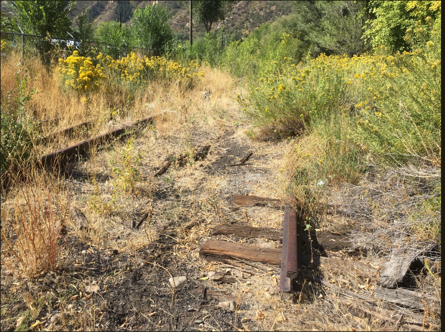
Southwestward view of the east branch of the wye a few steps from the previous location, where the remnants of a track are in the foreground and one track splits into two in the upper left.
