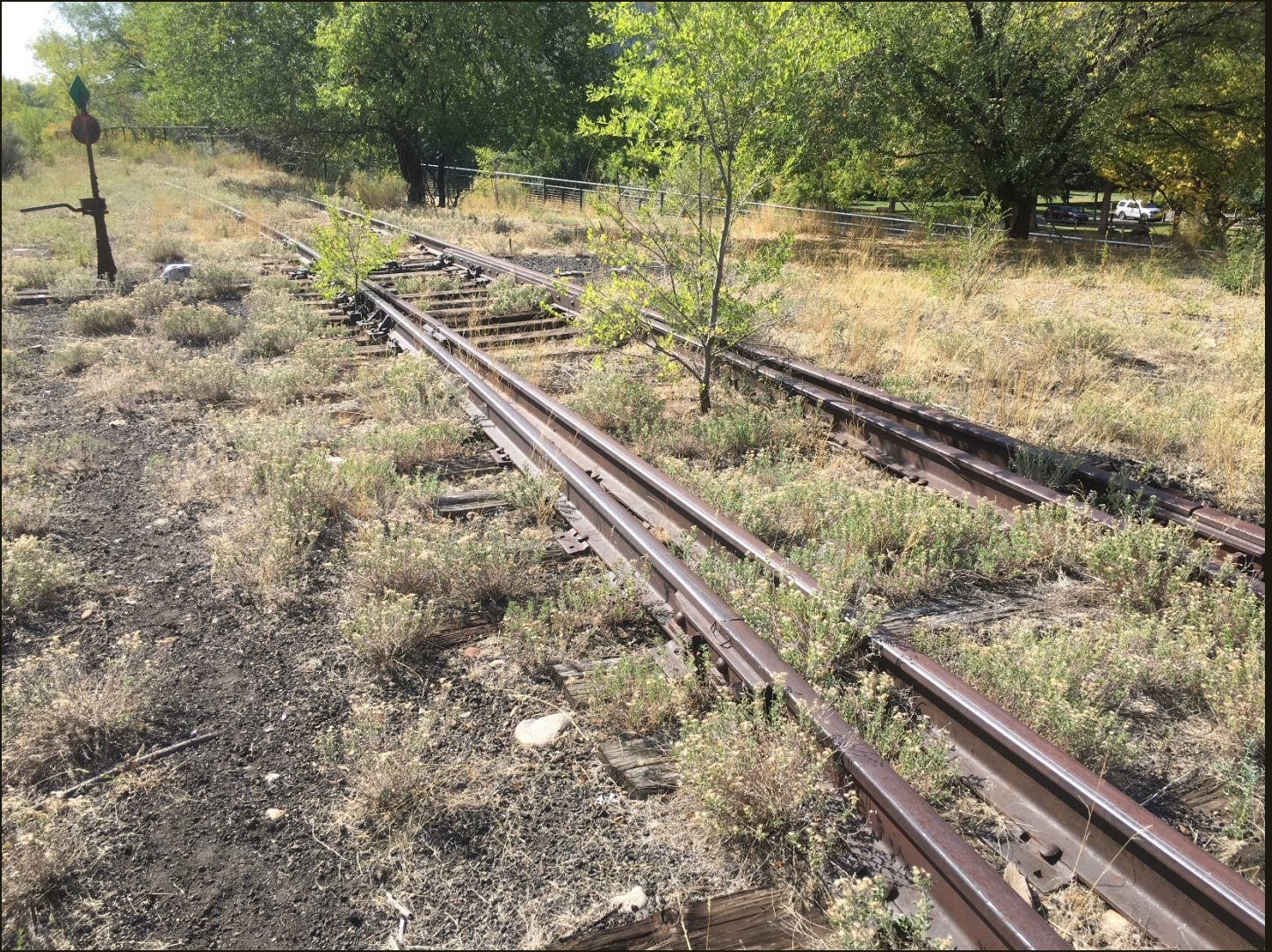
Southward view 100 feet south of the previous location at the south tip of the wye, where the east and west branches of the wye converge to the single track to Aspen. The fenced trail to the right is the Rio Grande Trail. At this point and for 1,500 feet to the north to the Colorado River, the Rio Grande Trail is not on the railroad grade (to avoid the wye).
