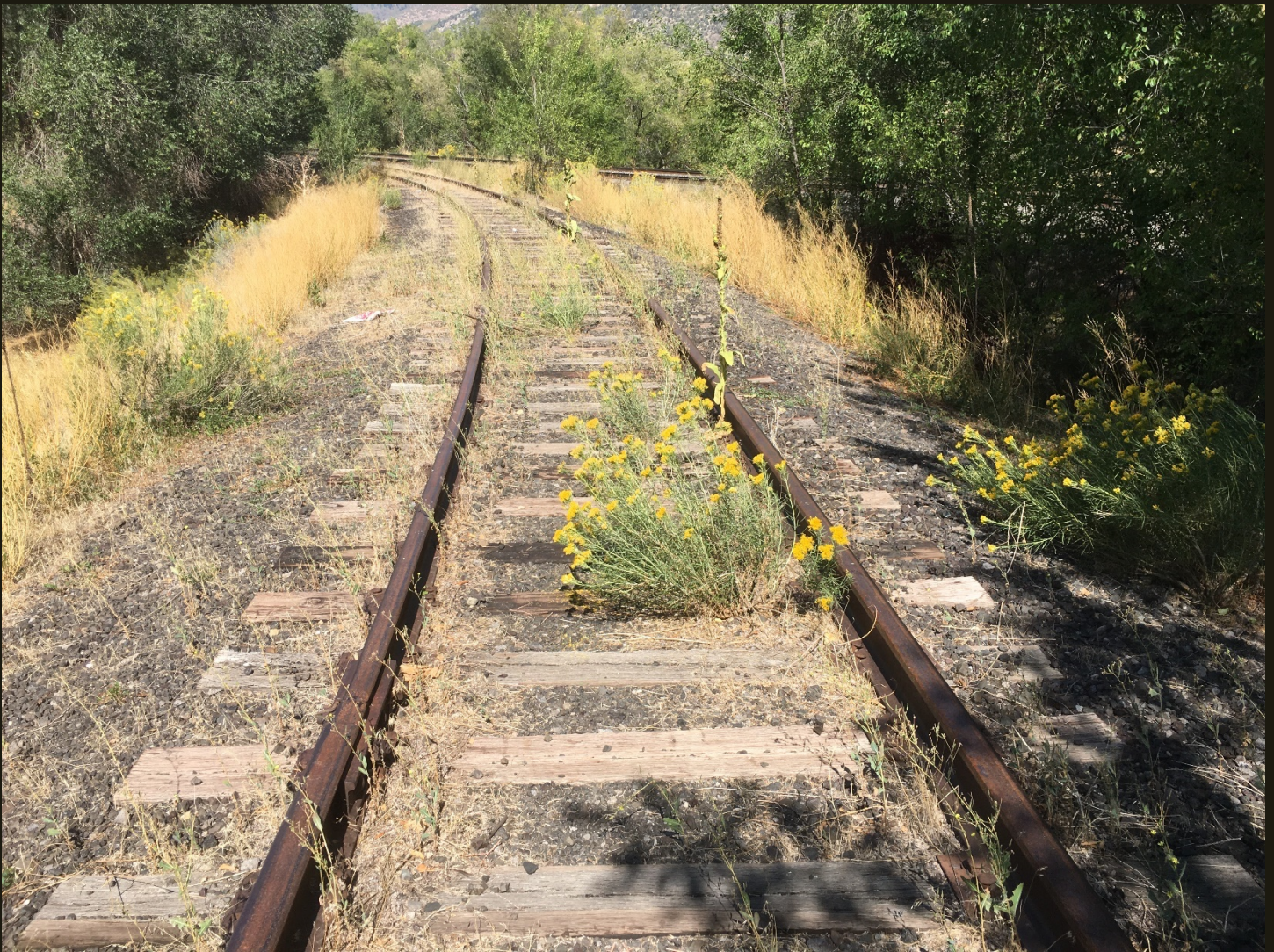
Northwestward view of the west branch of the wye 200 feet northwest of the previous location. The mainline in the distance is the 1967 realignment of the D&RG (1889n) to connect the D&RG Aspen Branch (1887n) to the abandoned CM (1888) grade. The 1967 realignment involved about one mile of new right-of way to connect the D&RG Aspen Branch (1887n) to the CM (1888) and is not shown separately on the Southwest Railroad History Map.
