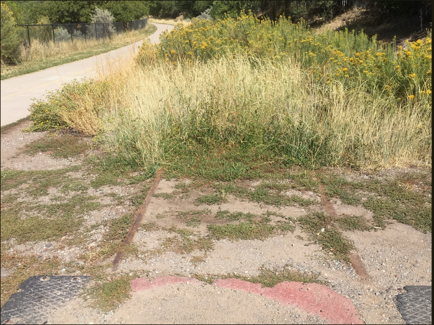
Northward view of the D&RG Aspen Branch (1887n) and Rio Grande Trail 1,000 feet south of the previous location. The tracks have been cut for installation of a utility vault.
