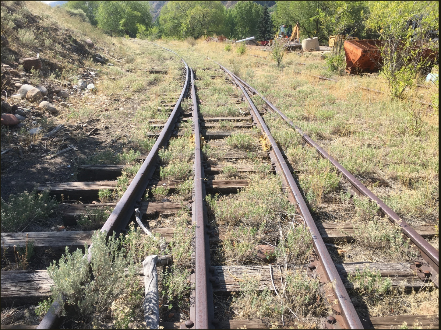
Southward view 300 feet southwest of the previous location. The tracks in the foreground are on the east branch of the wye and converge to a single track at this location. The overgrown track on the right is the west branch of the wye.
