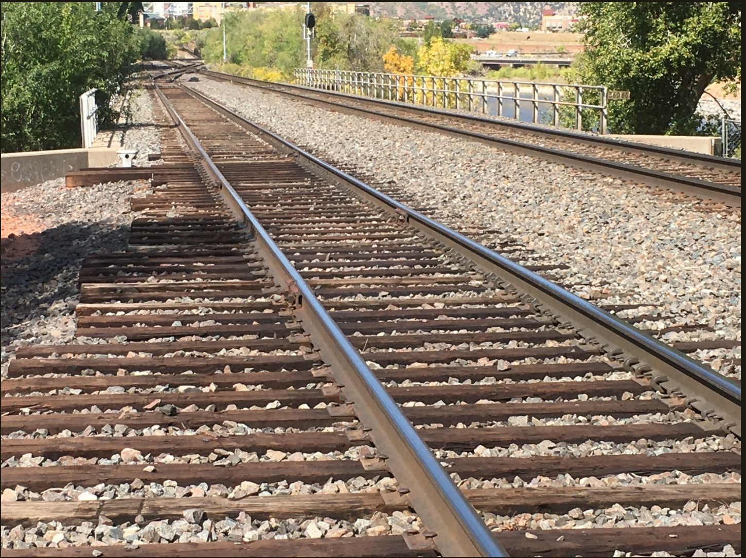
Westward view of the 1967 realignment to connect the D&RG Aspen Branch (1887n) to the CM (1888). The bridge carries the tracks over the Roaring Fork River, which flows into the Colorado River in the upper right of the photo. Just on this side of the bridge are two long ties that once served as the base of a switch to connect the west branch of the wye to the bolted-rail siding. The welded-track mainline is on the right and an additional siding splits off the mainline on the other side of the bridge. It is hard to tell exactly where the 1967 realignment intersects the original CM (1888) grade.
