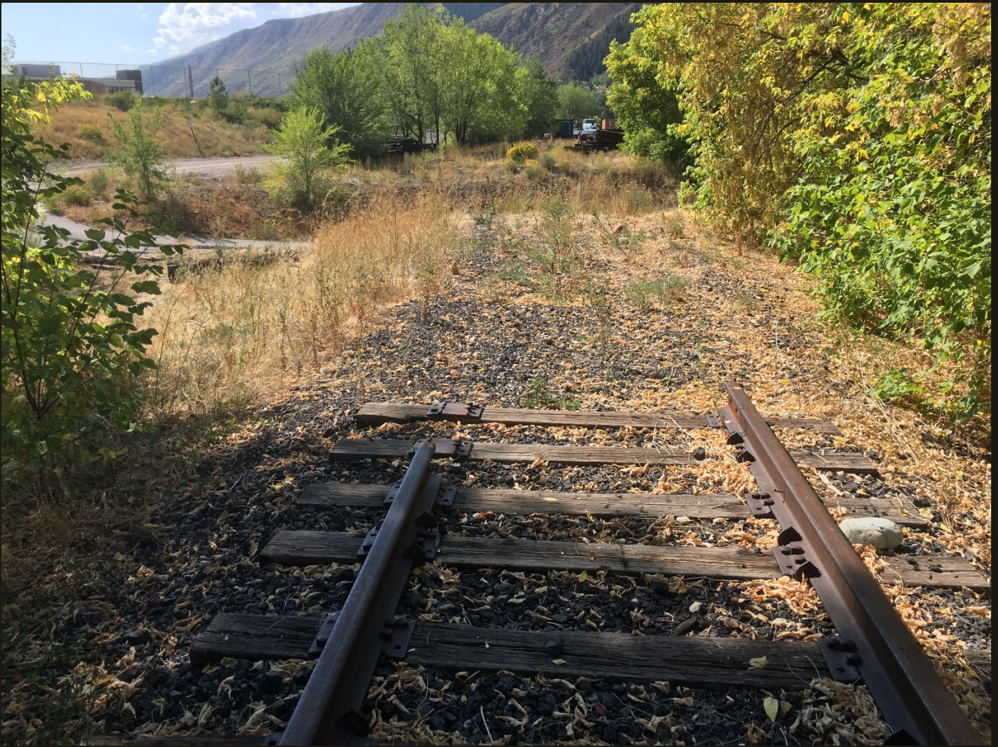
Southward view of the west branch of the wye for the D&RG Aspen Branch (1887n) across 8th Street from the previous location. A 1927 topo map shows a branch line that started at the north end of the current west branch of the wye, which at the time was the mainline to Aspen, that branched southwestward on the current alignment of 8th Street and continued west over the Roaring Fork River to the CM (1888) alignment, where a half mile of track was in place apparently for D&RG car storage. A 1961 topo map shows that branch line replaced by the current 8th Street, seen here. The east branch of the wye (this location) was built in 1967 and apparently had a level grade crossing of 8th Street, which was apparently regraded and cut the tracks during the 1995-2006 abandonment of the Aspen Branch.
