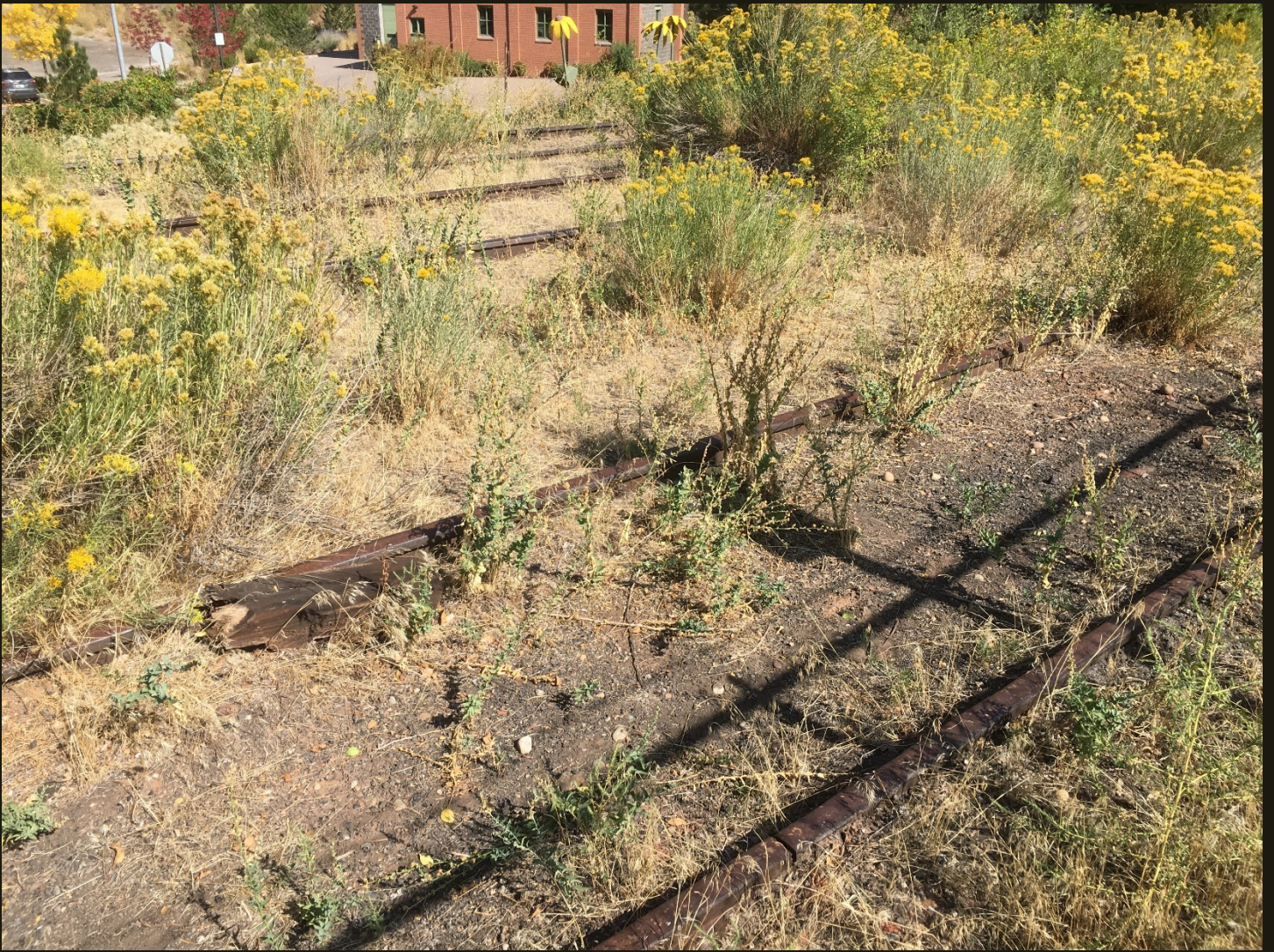
Northwestward view of the three tracks of the east branch of the wye for the D&RG Aspen Branch (1887n) a few steps from the previous location.
