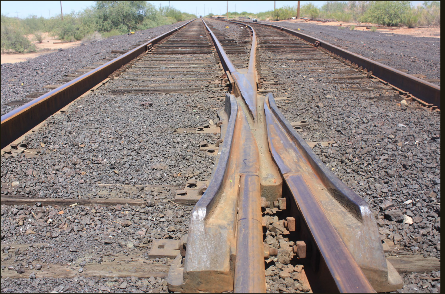
Same view as previous, with close-up of the siding switch cross-over. Note all bolted track.
