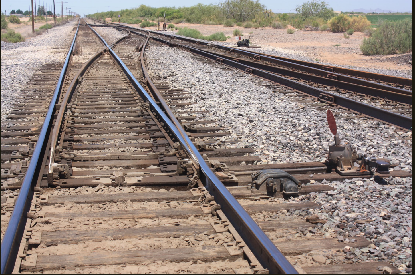
Same location as previous photo, looking north; from left (west) to right: the shiny 1924 SP Phoenix connection, the P&E mainline, and the switch to the rusty P&E siding. The double track in the distance extends one mile north from Magma, where the P&E mainline merges with the SP line.
