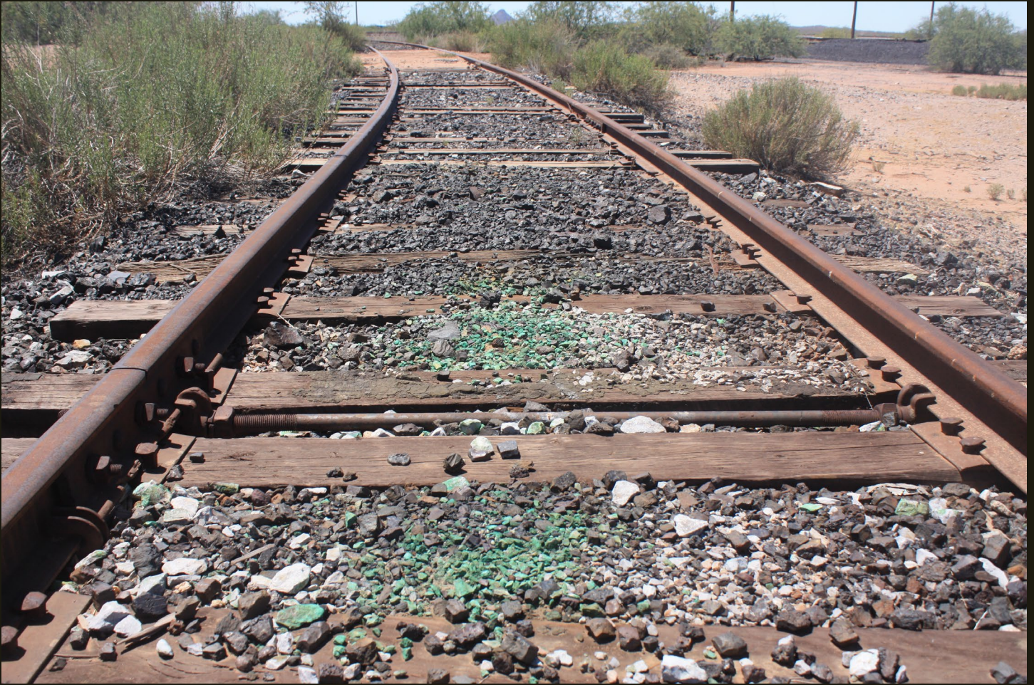
A closer look at same location as previous shows some green copper ore that fell onto the tracks of the south leg of the MA wye at Magma.
