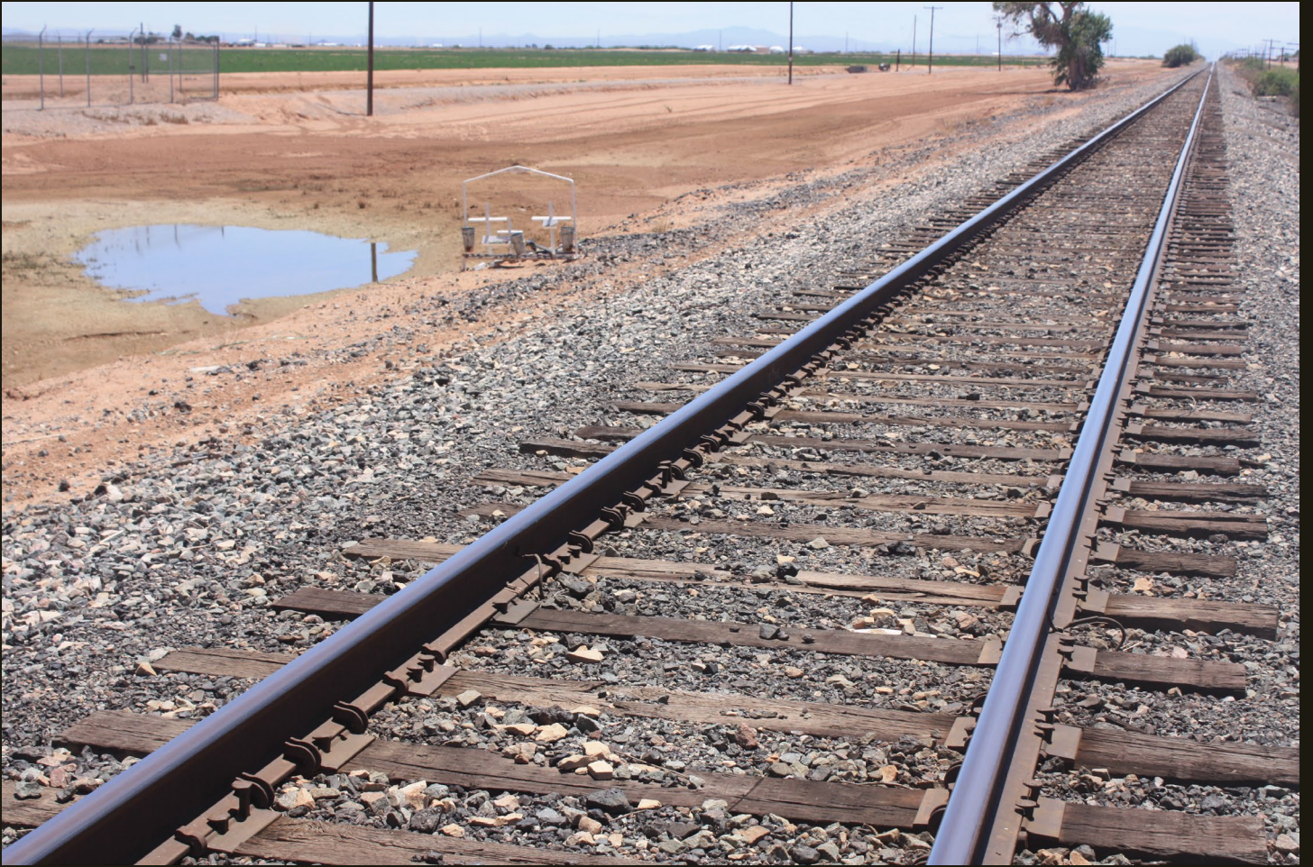
Southward view 2 miles north of Magma, where the 1924 SP Phoenix connection is built on the 1904 P&E grade.
