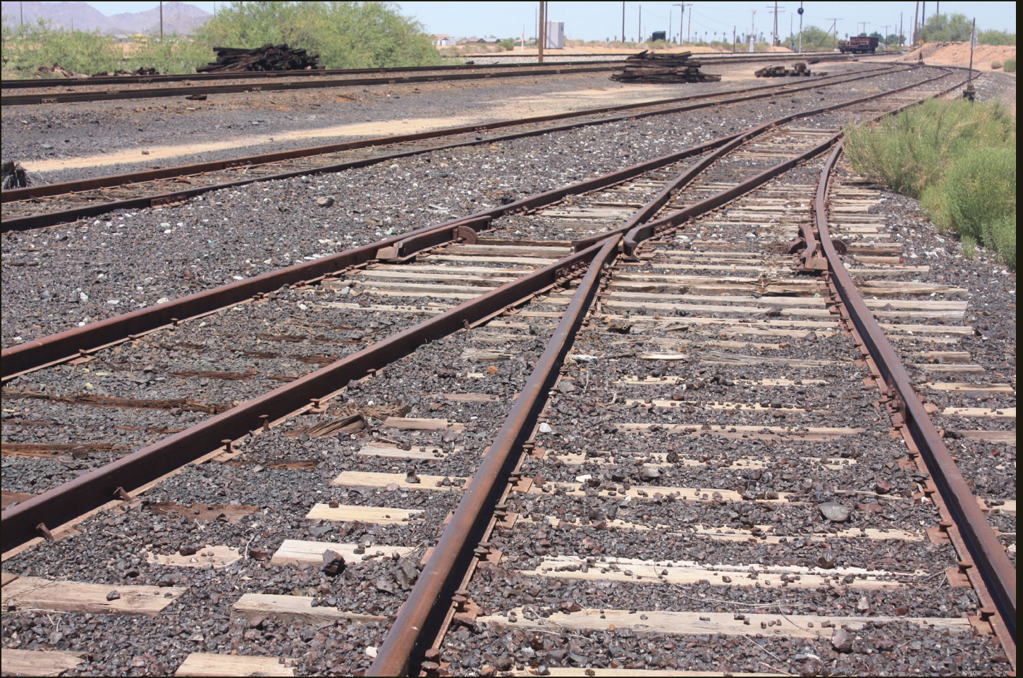
Northwestward view of the northern leg of the MA wye, where it joins the MA siding, with the second MA siding and the P&E siding and mainline to the left (west). Note the same stored car we've been seeing on the P&E mainline. Note also in the distance another track on lighter gray gravel ballast, the Southern Pacific (1924) line discussed below.
