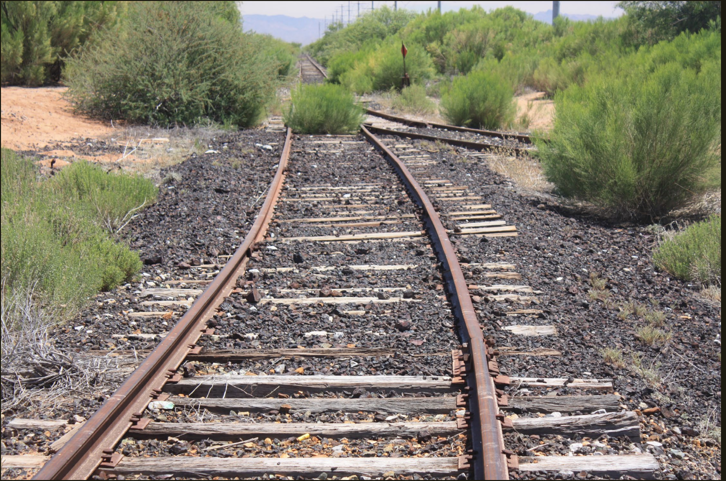
Northeastward view of the apex of the MA wye and the beginning of the MA, built in 1915 as a narrow gauge road.
