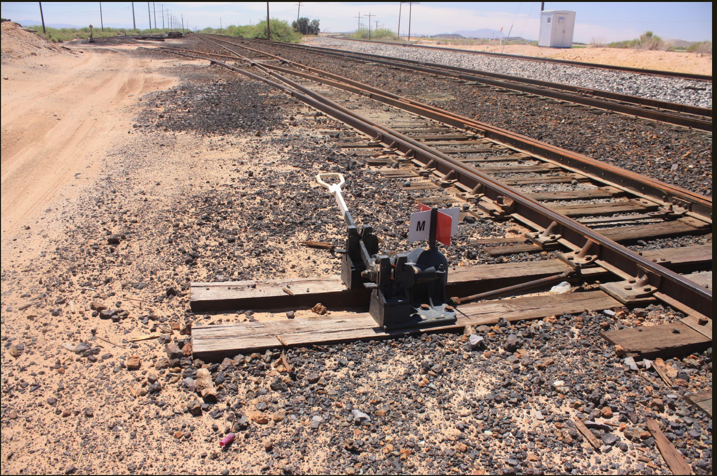
A little farther north, looking south at the switch where the MA siding joins the P&E siding. The switch with the yellow diamond sign in the left distance is where the two MA sidings converge to a single track. The P&E mainline is to the right (west) of the P&E siding and a new line is at the far right with fresher-looking gray granite ballast. That line is the last chapter in the railroad history recorded at Magma, the Southern Pacific's 1924 Phoenix connection.
