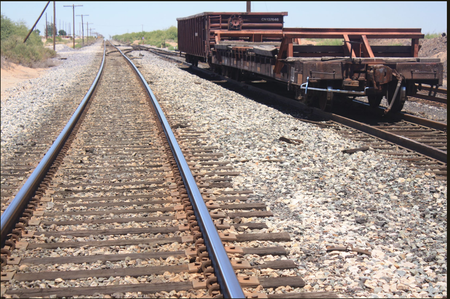
Same location as previous photo, looking north; from left (west) to right: the shiny 1924 SP Phoenix connection, the P&E mainline with the same stored cars, and the P&E siding.
