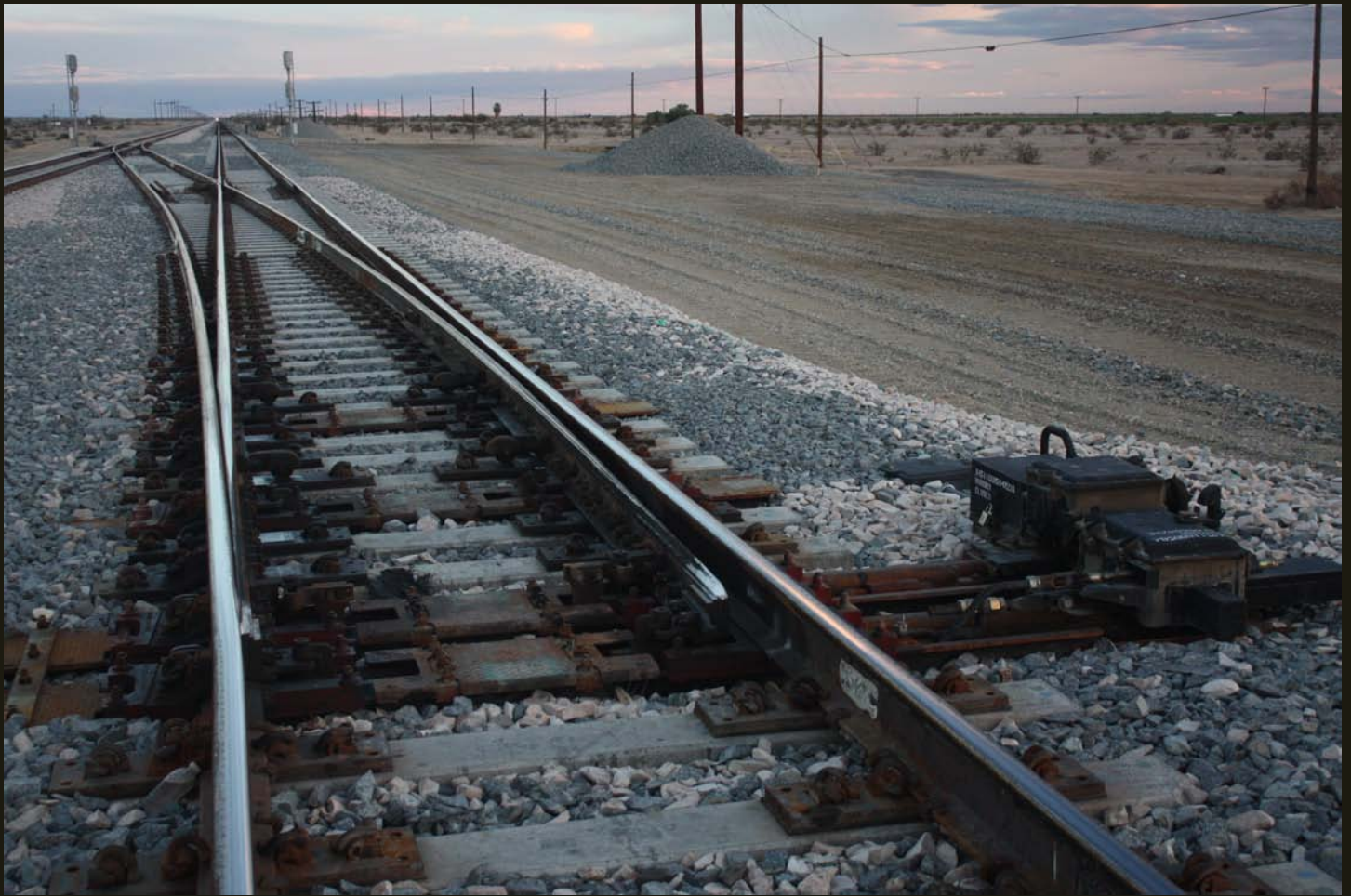
The SP mainline, built around 1880 through the Salton Trough, has two tracks with a cross-over just southeast of the Niland wye. The right track is older, with wooden ties except where this cross-over was built. The older line interchanges directly with the Inter-California line.
