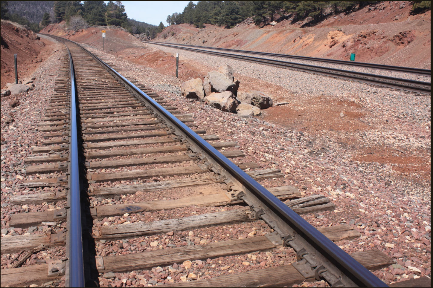
Westward view, same location as previous. The track in the foreground is the 1960 connector to the A&P (1883) and the SFP&P (1895) and the two tracks on the right are the AT&SF (1960).
