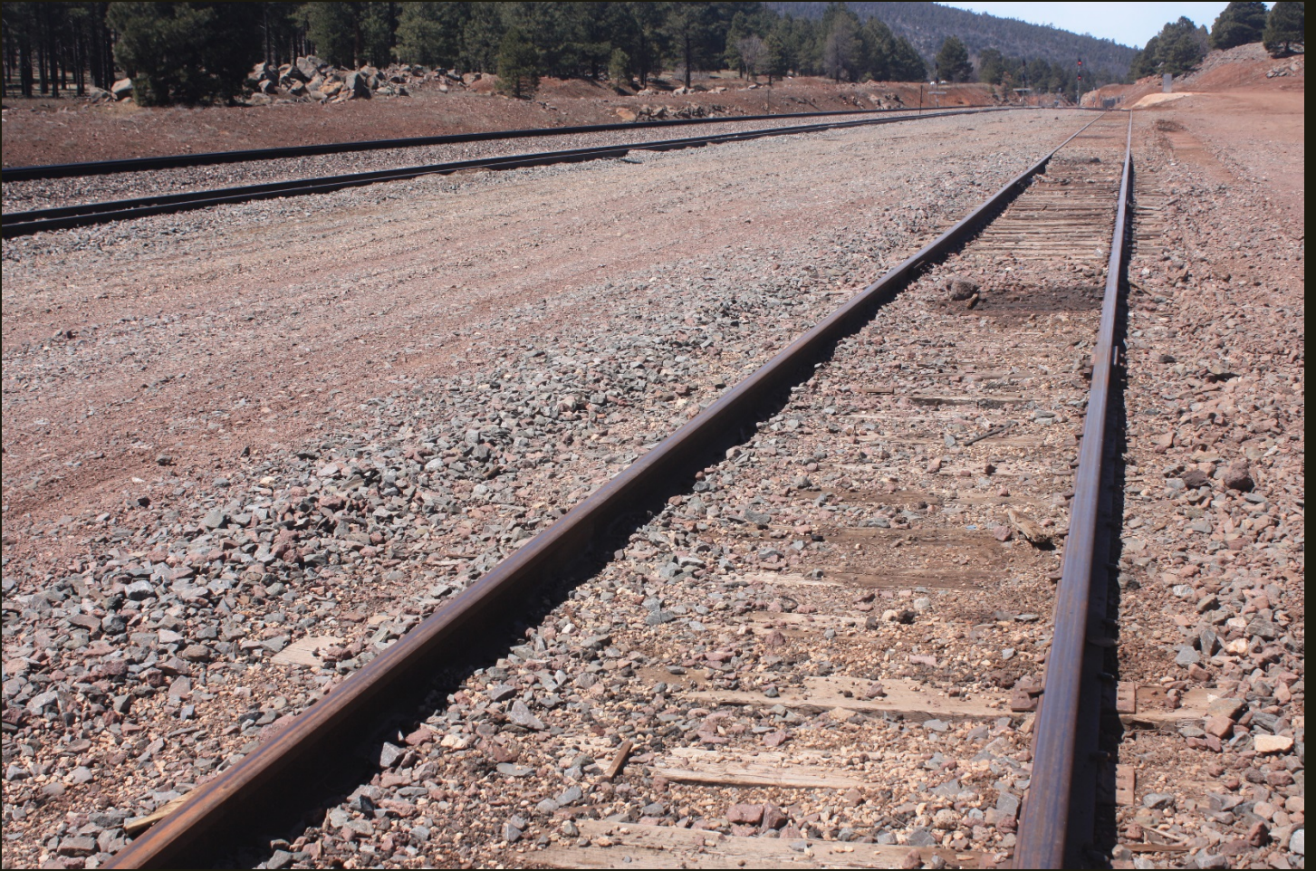
Westward view of the AT&SF (1960) same location as previous. The track in the foreground is the outer siding, the track to its left is the siding that connects to the mainline at both ends, and the higher track to its left is the mainline, which is a double track (but only one track is visible in this view).
