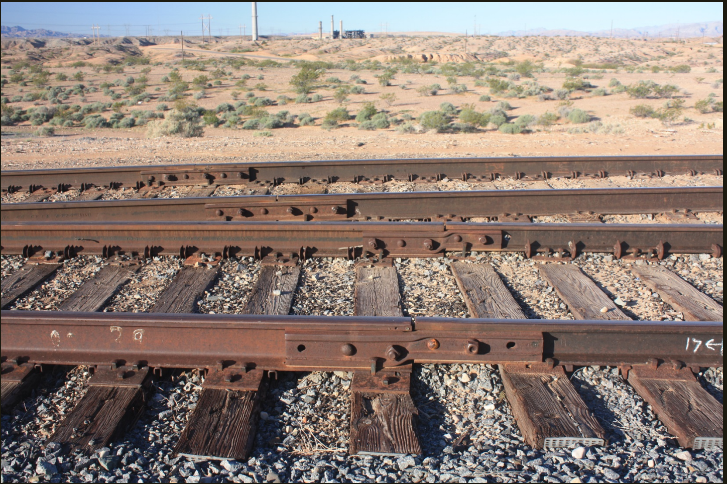
Southwestward close-up of the converging tracks at the tip of the wye. Note that the bracket for connecting the rails is bent to accommodate rails of two different weights, the rail to the right being the lighter of the two rails.
