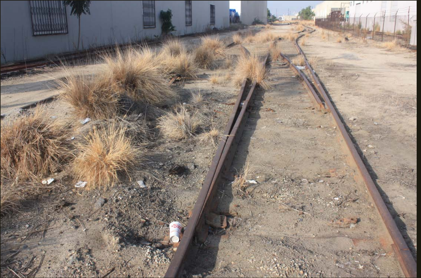
Overgrown and rusty LAJ spur.
