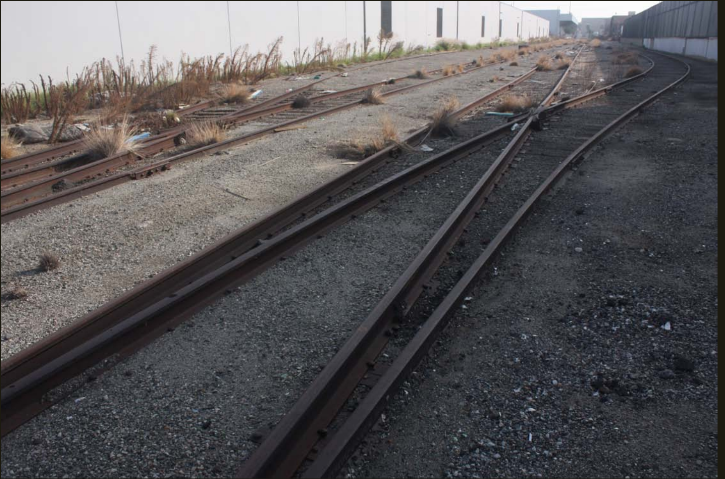
Another overgrown and rusty LAJ spur and sidings.
