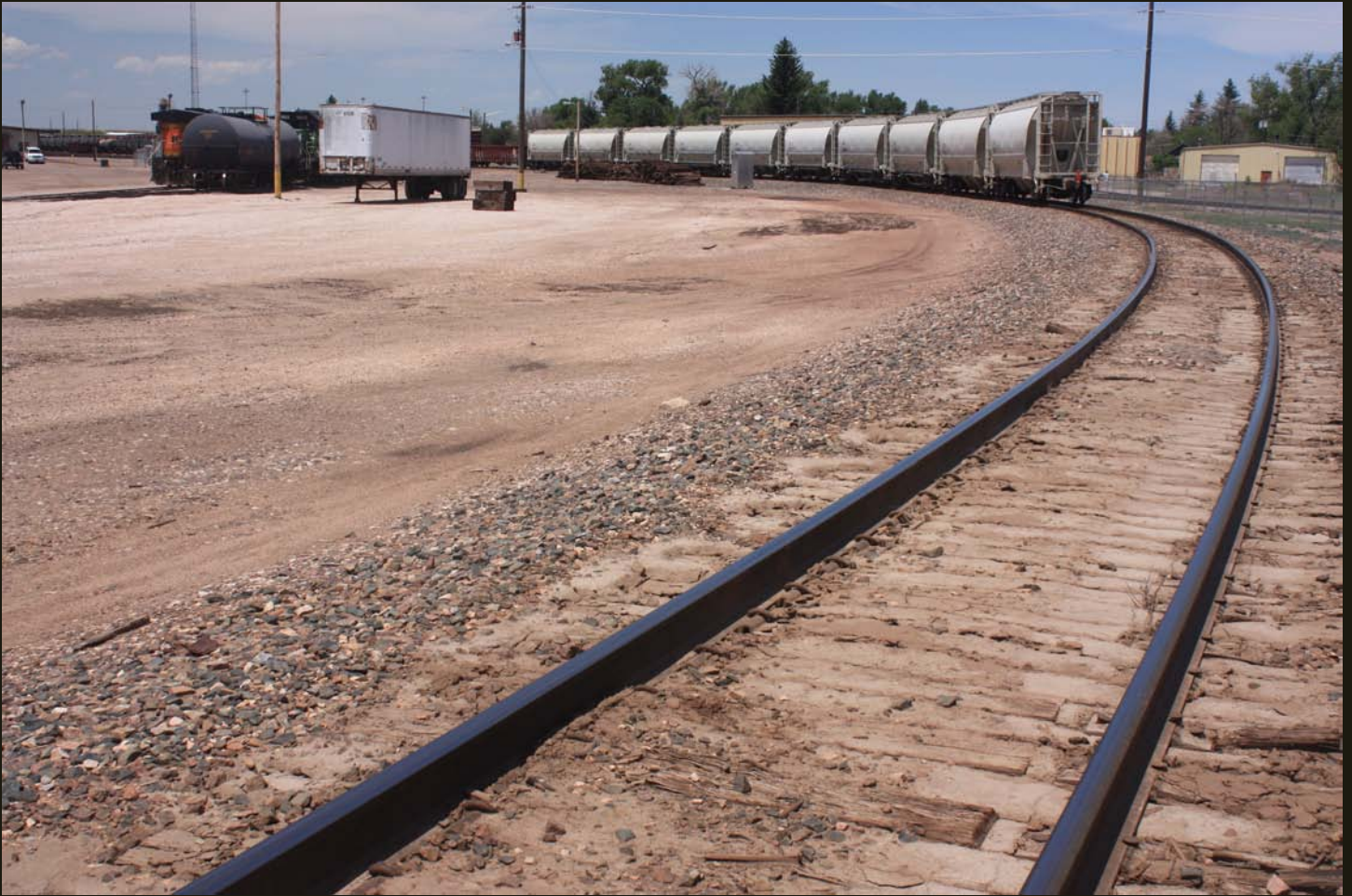
The C&N rails south of the north Cheyenne wye (to downtown Cheyenne and the C&N connection with the UP) are used for car storage.
