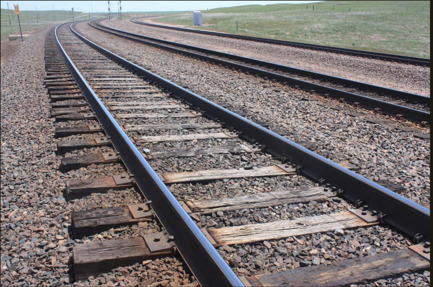
Eastward view of the UP mainline 10 miles west of Cheyenne. The double track on the left is the UP mainline and heads down to Cheyenne on Crow Creek. The track to the right is a cutoff that heads up and southeast to connect with UP single track built in 1918 located about a mile to the south of this location; the 1918 track connects to the DP line south of Cheyenne.
